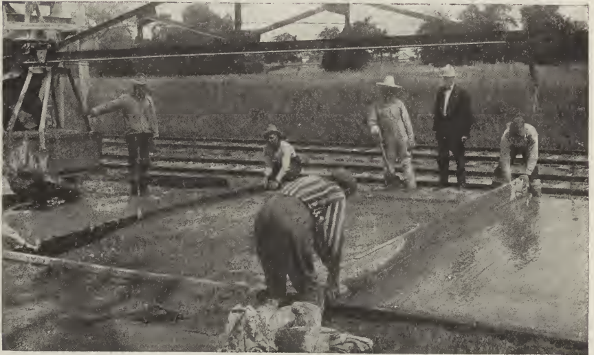
FIG. 36.—Near view of curved strike board for giving the crown to the pavement, showing also concrete bucket, mixer, boom, and steel expansion joint in place.
