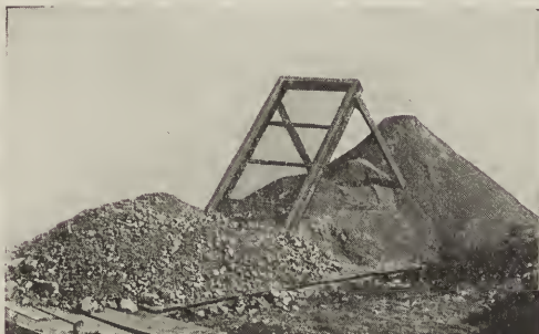
FIG. 11.—A slanting screen can be made to separate the sand from the coarse material in bank-run gravel, making possible a great improvement in the quality of the concrete produced.
