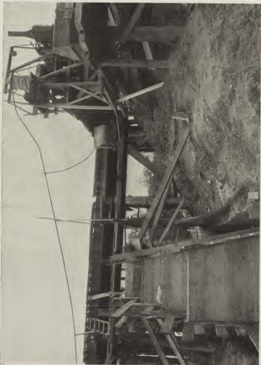
Fig. 20.—View showing method of transporting and placing concrete for railroad bridge abutments.
