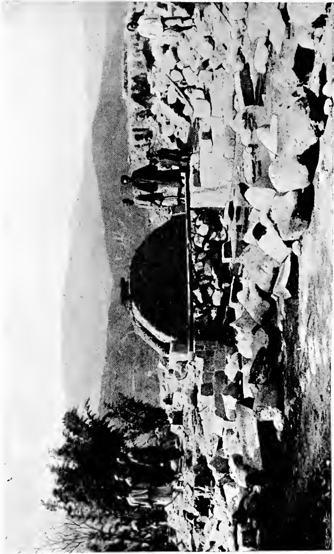
BUILDING A NEW BRIDGE OUTSIDE THE EAST GATE OF NANTIEN, FAR WESTERN CHINA.
