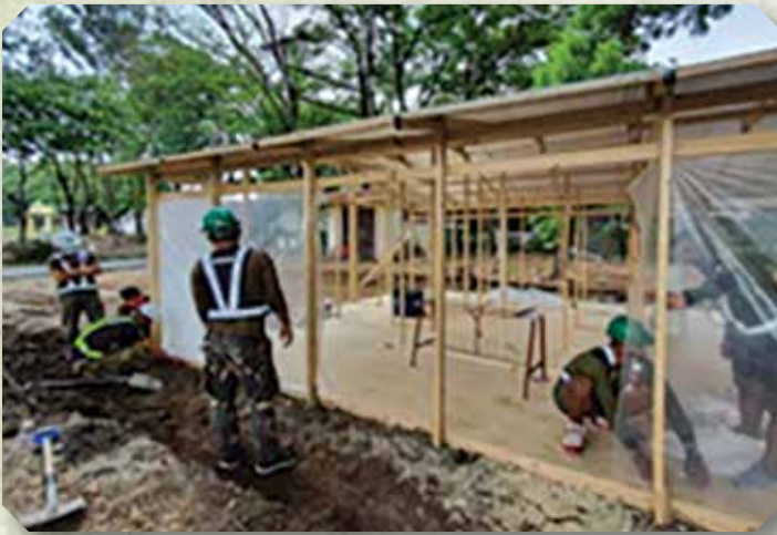
Construction of Emergency Quarantine Facility (EQF) of NOLCOM Hospital at Camp Aquino Tarlac City.
