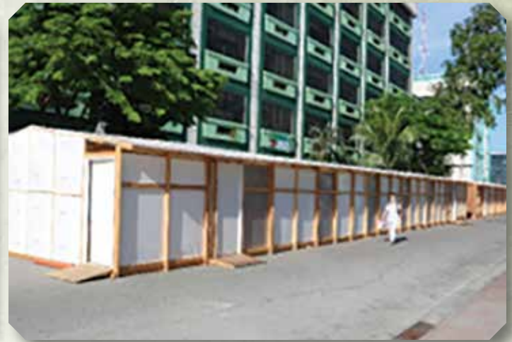
Completed three units Emergency Quarantine Facility (EQF) at Amang Rodriguez Memorial Medical Center, Marikina City.
