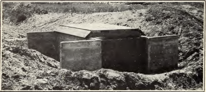
FIG. 2.—RADIAL DELIVERY GATE, TURLOCK IRRIGATION DISTRICT, CALIFORNIA.
