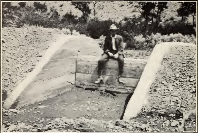
FIG. 1.—WASTE GATE ON LAKEVIEW IRRIGATION CO. CANAL, WYOMING.
