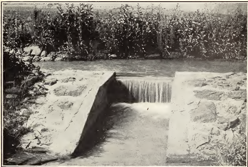
FIG. 2.—WASTE GATE ON SMALL LATERAL, YAKIMA PROJECT, UNITED STATES RECLAMATION SERVICE.
