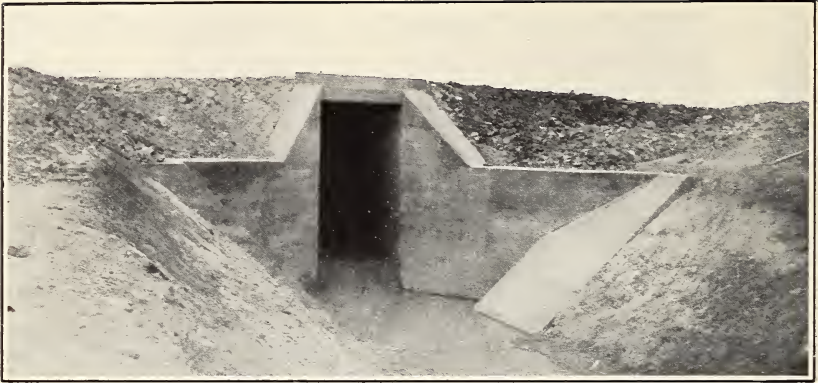
FIG. 1.—HEADGATE, LOW LINE LATERAL, ROCK CREEK CONSERVATION CO., WYOMING.
