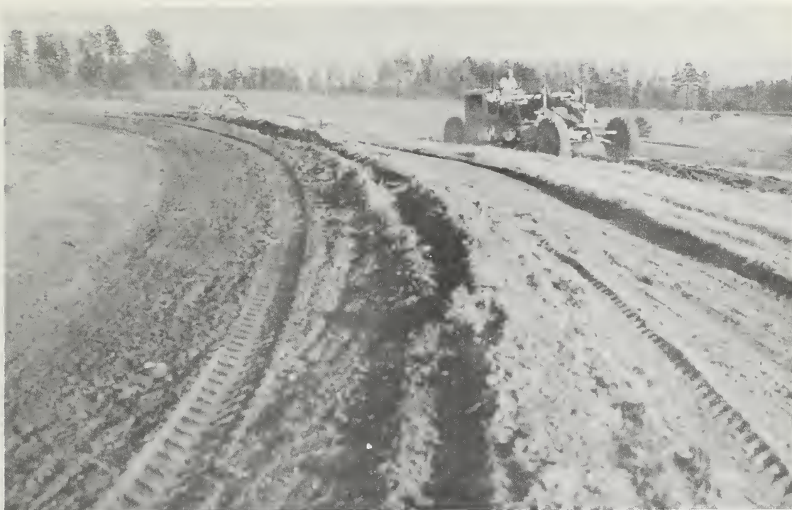
This grader is constructing a terrace in Rutherford County, leaving a ridge and channel at left to convey water. Apple trees will be planted along the ridge of the terrace.
