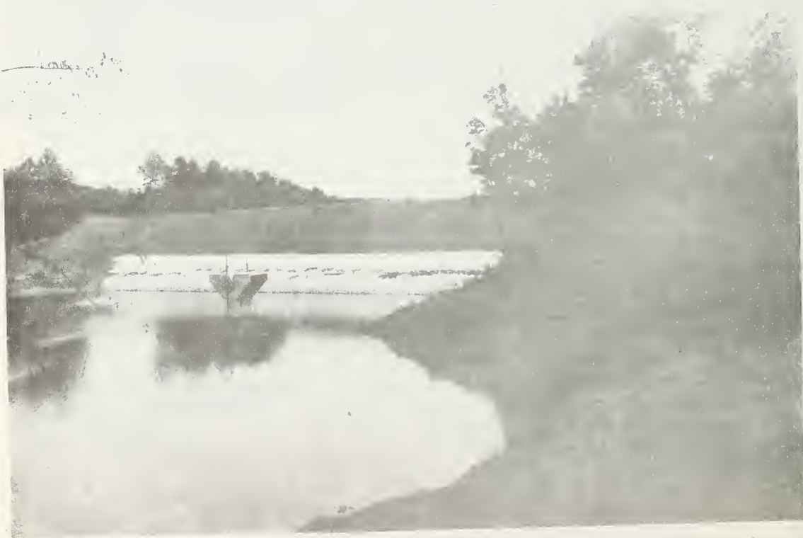
Another view of the same structure showing the dam and concrete riser.
