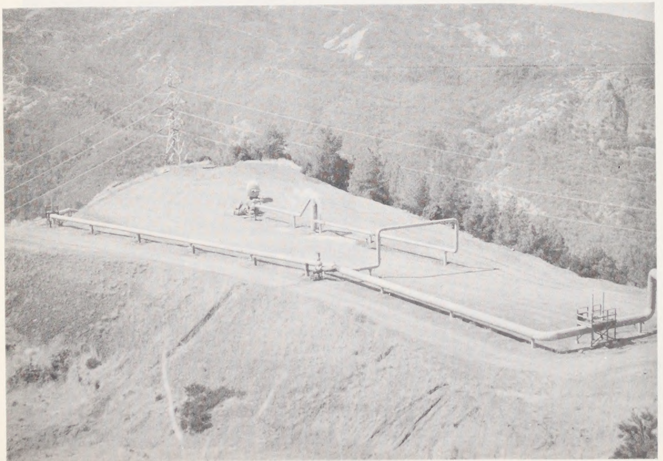
PIPELINES AT THE GEYSERS
