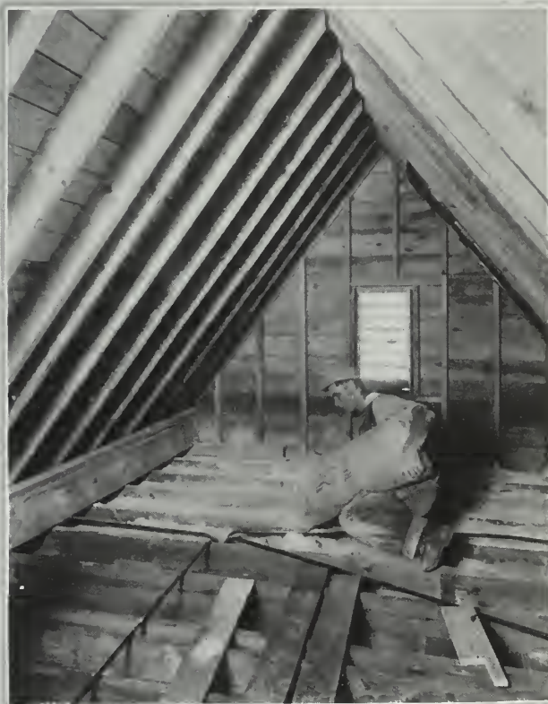
Dry-fill insulation installed between attic joists provides an insulating blanket over the rooms below, and saves the bulk of the heat that is lost from the average uninsulated dwelling. Such insulation also keeps the rooms below cool in summer
