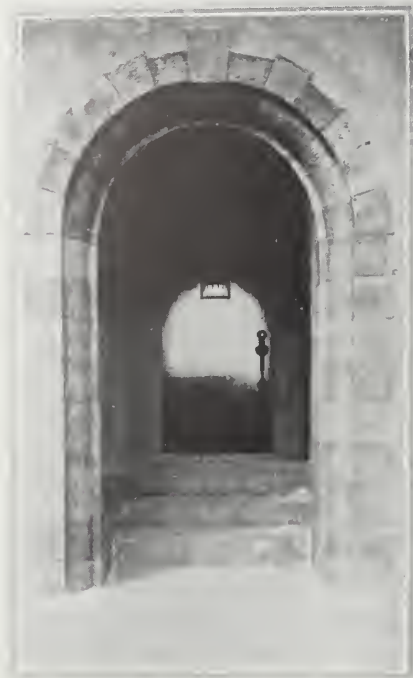
Detail of the front entrance doorway with its "stonework" facing developed in stucco and colored in browns and greens to give contrast. The effect of the two arches is good
