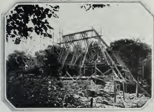
No very definite idea of final results can be gained from these pictures of the 1928 COUNTRY LIFE house in process of construction, but the
