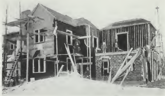
Illustrating the manner of applying cork board over sheathing as exterior insulation. Waterproof paper is applied over the insulating material, and furring strips are partly in place to receive metal lath for the finishing coat of stucco
