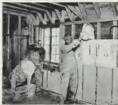
Applying the poured or cast type of insulating material, which when combined with water expands into a froth that sets in a rigid mass
