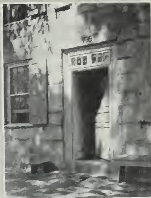
Entrance doorway to the original Sackett homestead, showing the date, 1799, carved on the lintel
