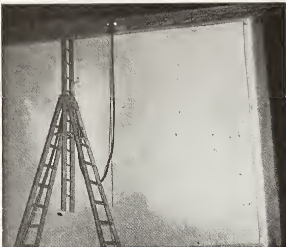
Setting up for mechanical screen resurfacing (above). The track starts at top and carries the spray gun (see detail view below) across the screen in downward steps.
