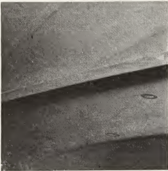
Details of the Paramount Tacna's auditorium ceiling, finished in finely corrugated plaster which controls reflection of screen light through the angle of the indentations. Screen light thus contributes to running illumination.
