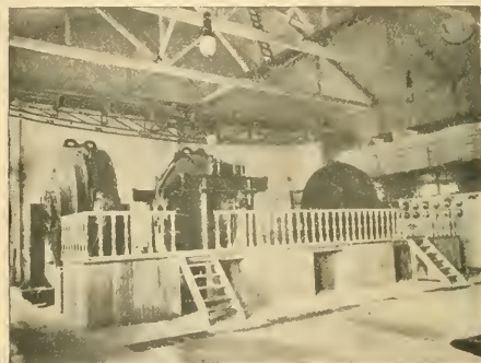
FIG. 4.—Photograph of three 500-kilowatt furnaces at Notodden.
