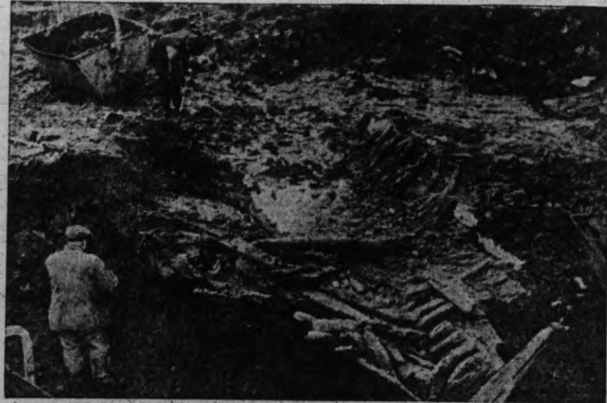
MAKES ITS NAILS WORK. —Dug for more than 100 years, the nails which were discovered recently by excavators on the site of the new New York Telephone Co. building. Hand-made nails held the wood together.
