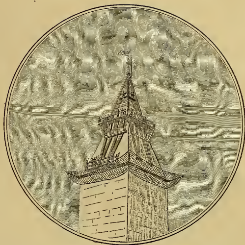
STAGING AT THE TOP OF THE MONUMENT DURING THE WORK OF COMPLETION.
