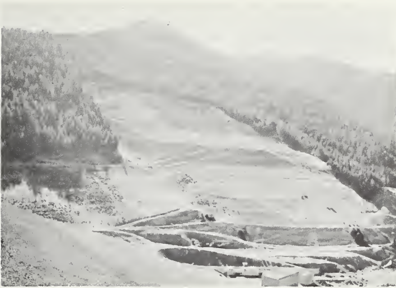
Landslide at toe of Trinity Dam on the east abutment. Treatment measures on slide include benching at intervals and a system of drain lines and collector pipes.
