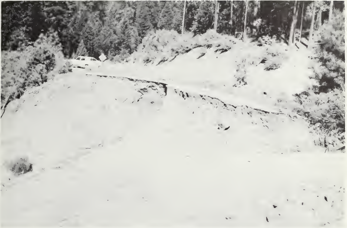
Landslide damage to a seventy-foot high road fill.
