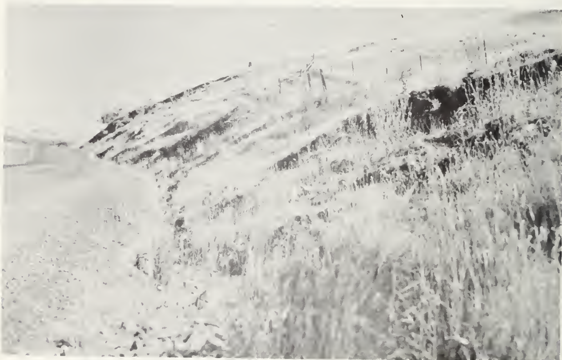
Eroding roadside ditch causing slides on the roadcut.
