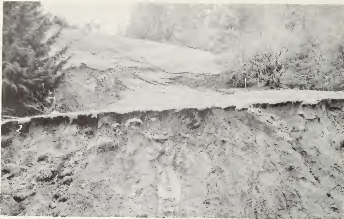
Land slippage and roadside erosion. SCS PHOTO 3-2220-10
