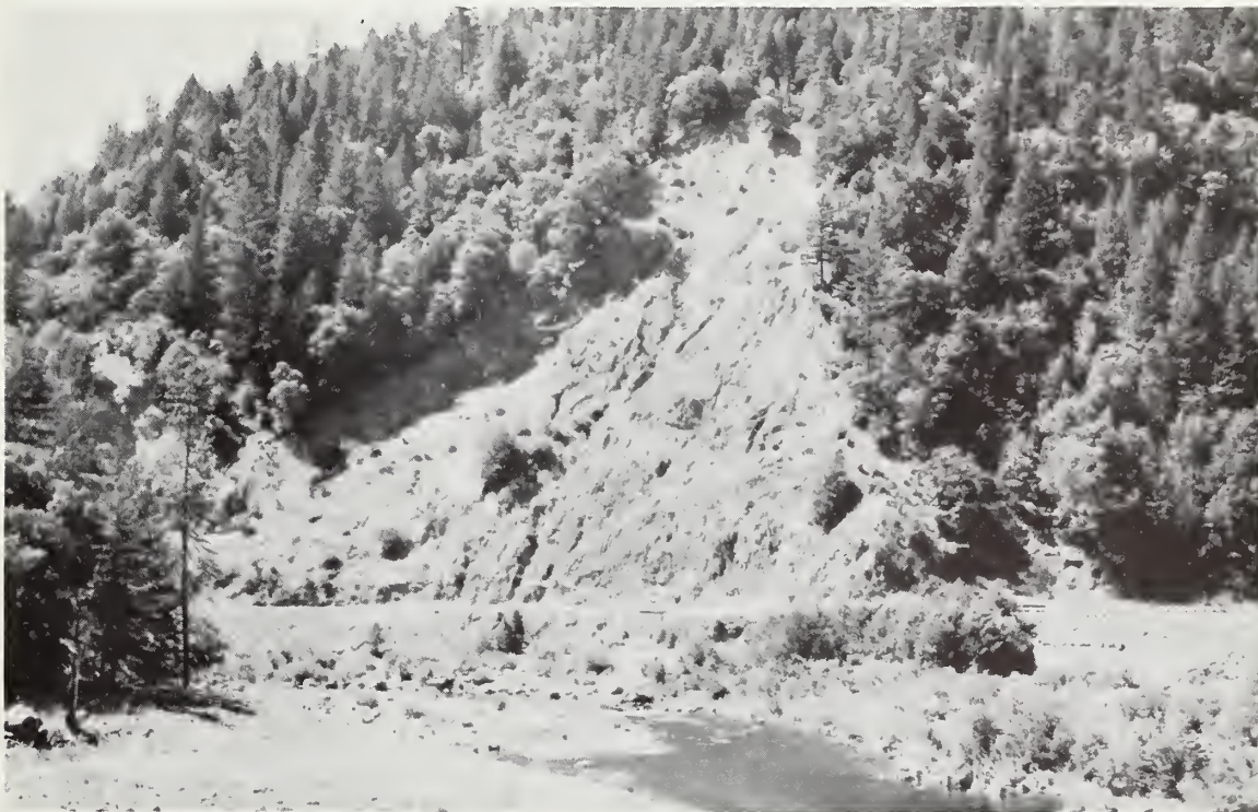
Landslide in road cut on State highway 299 along the Trinity River.
