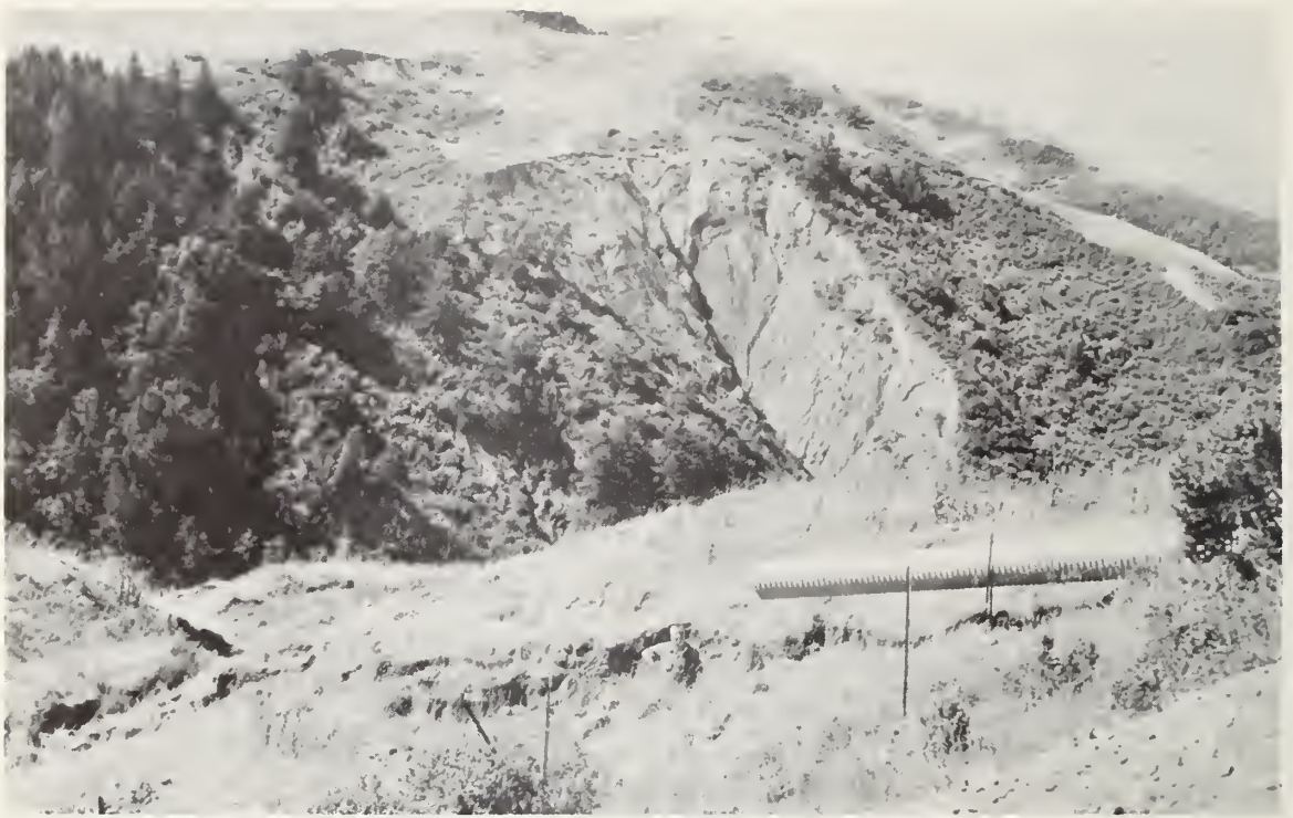
Road culvert outletting above ground on unstable soil causing erosion. Landslide on far hillside.
