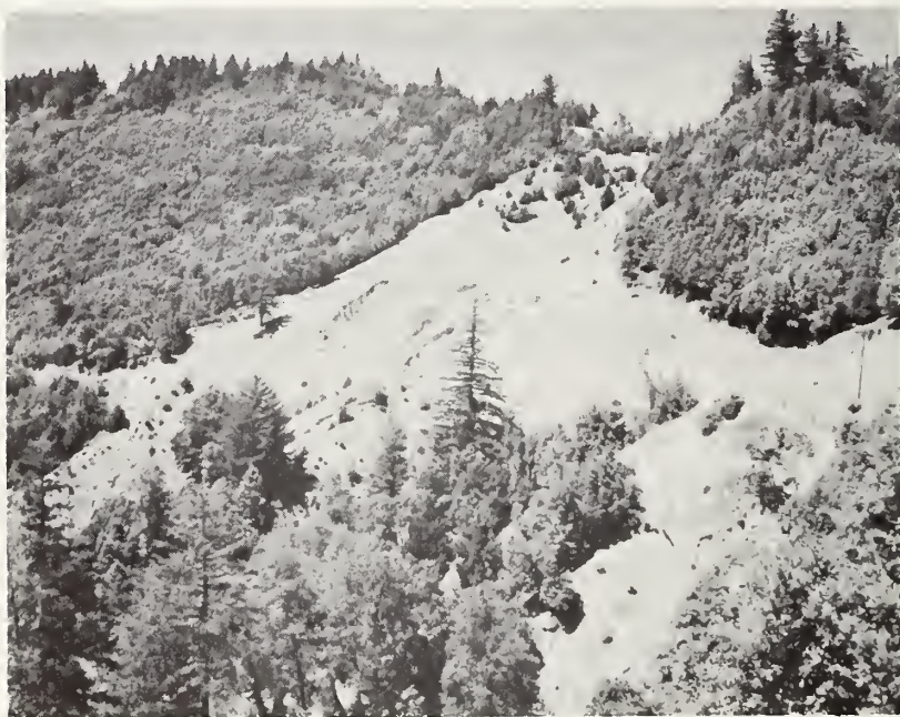
Landslide badly gullied from poor drainage conditions. Drainage pipe on the slide ends 25 feet above road and is causing gully.
