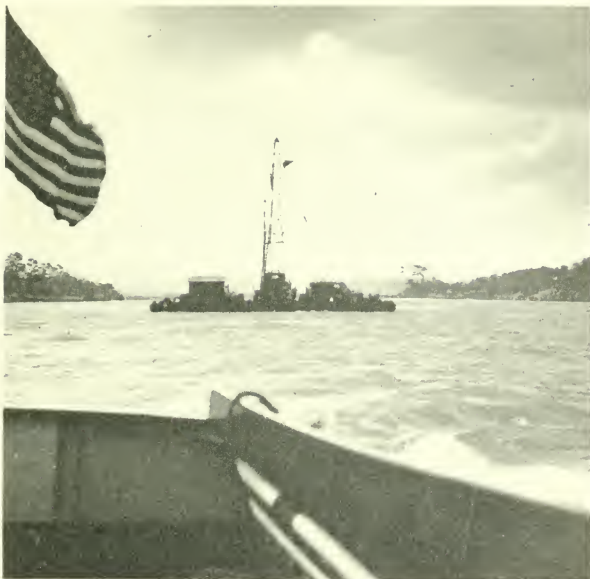
1. Test drilling and blasting at unprecedented depths of 135 feet below water surface are being carried out from a barge plant in the approach to the Third Locks Cut on the Atlantic side.
