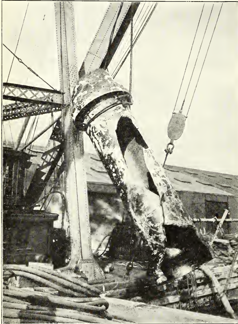
HOISTING THE DAMAGED WATER-PIPE ABOARD THE FLOATING DERRICK
