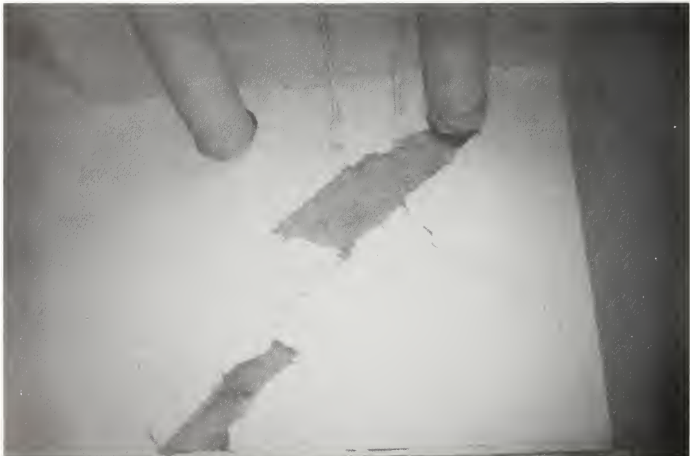
Figure 4.4.27 Cracks in the stair-well shear walls of the Osaka Airport Administration Building.
