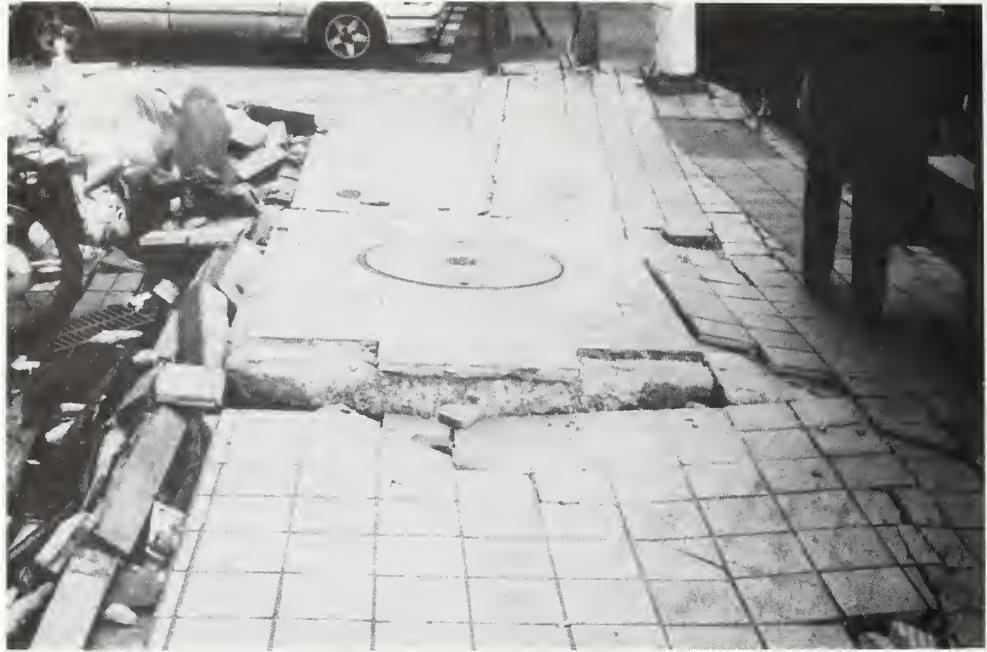
Figure 5.5.8 Subsidence around manhole can damage conduit and trunk lines.
