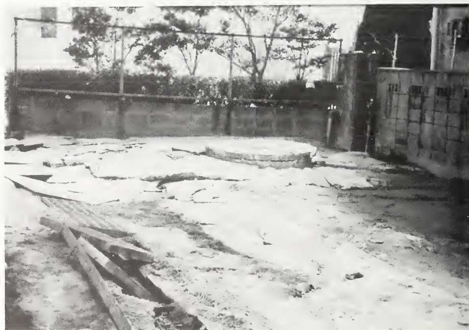
Photo 25 Manhole floated as a result of liquefaction near the wastewater treatment plant.
