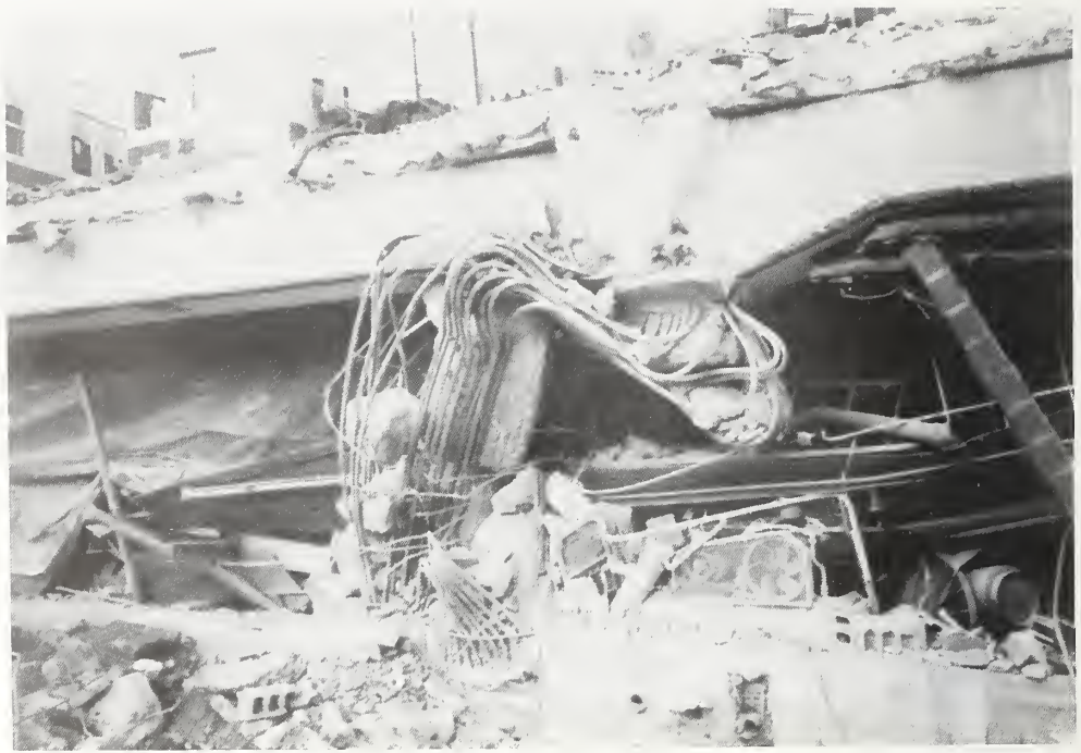
Figure 4.3.9 Failed column at Higashi - Nada - elevated rail yard.
