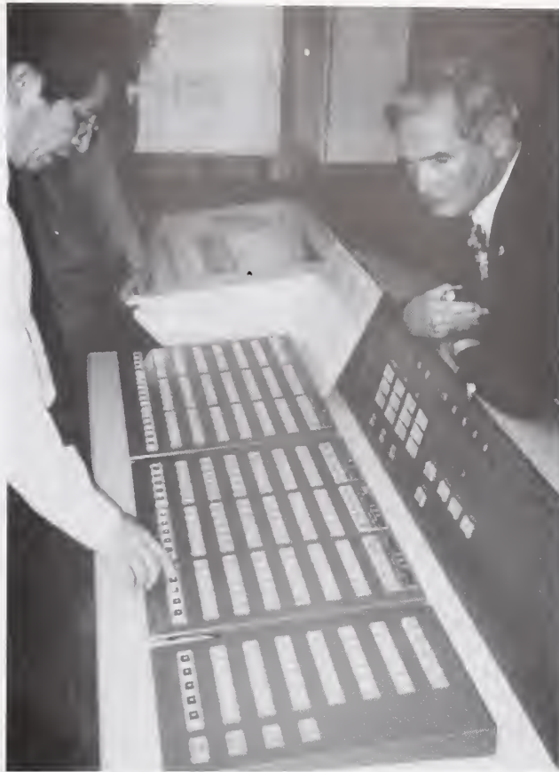
Photo 6 Control Panel for earthquake valves to provide flexibility to control automatically or by operations staff in Okuhirano Control Center.
