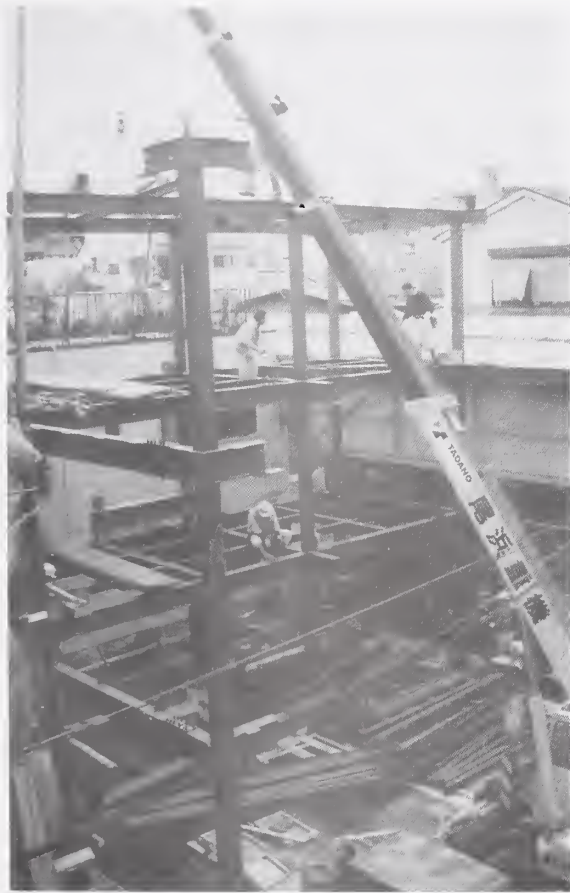
Figure 3.5.1 Typical modern 3 story new steel frame building being erected near Hanshin Expressway #3 east of Kobe. Columns are pre-fabricated so that no field welding is required.
