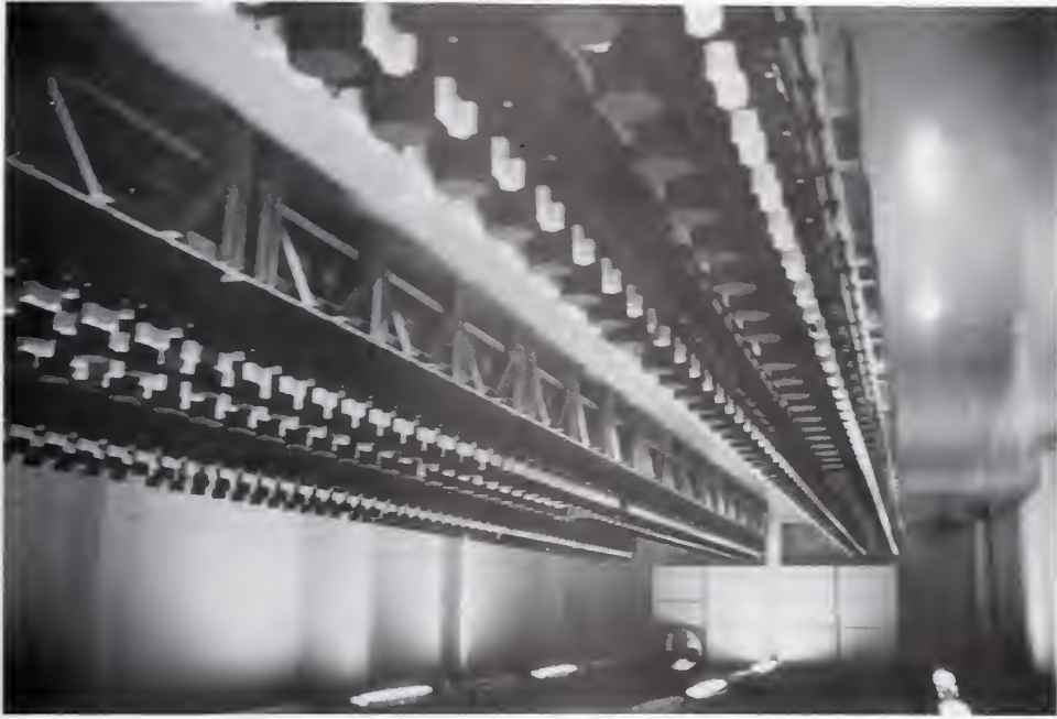
Figure 4.4.19 Very long battery string on low slung battery racks provides emergency power.
