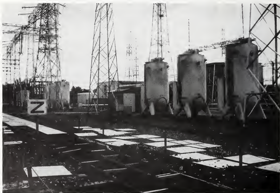
Figure 5.4.26 Bulk-oil circuit breakers with the bushings removed to replace damaged units at other sites.
