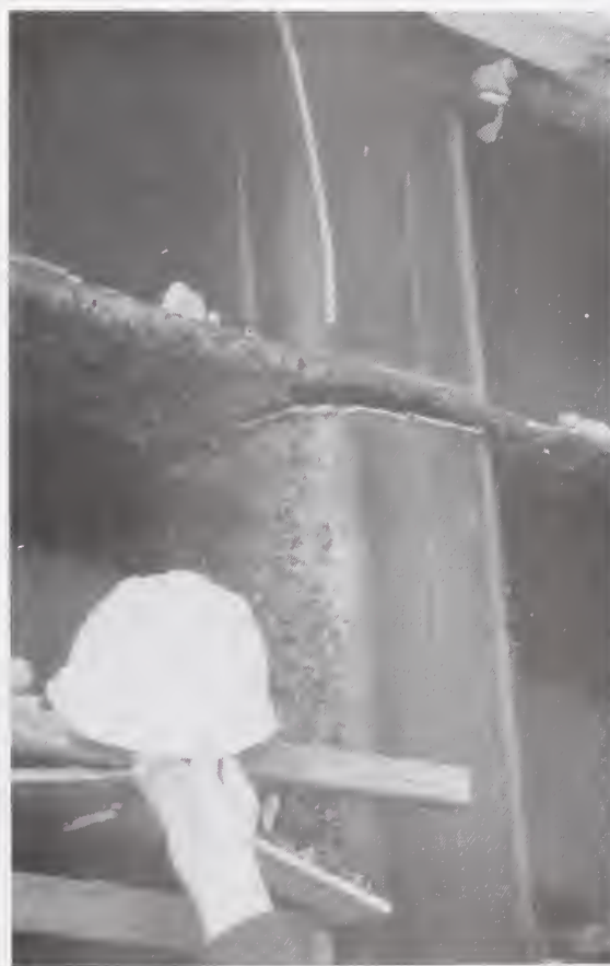
Figure 3.5.21 Closeup photo of column fillet weld failure in the Nairo Hiro building .
