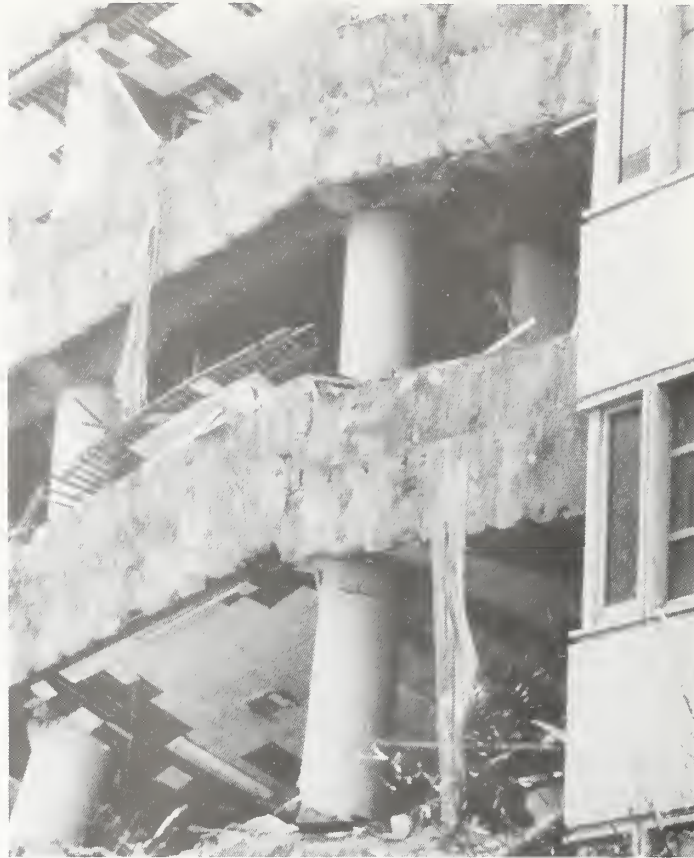
Figure 3.4.13 Strong beam-weak column failure.
