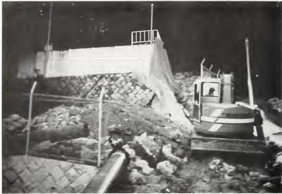
Photo 13 Broken lines to/from backwash tank at the Motoyama Water Purification Plant .
