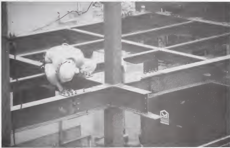
Figure 3.5.2 Field joint assembly of prefabricated steel frame structure east of Kobe using all high strength bolted connections. Beam stubs, approximately 0.5m in length, are shop-welded for quality control improvement.
