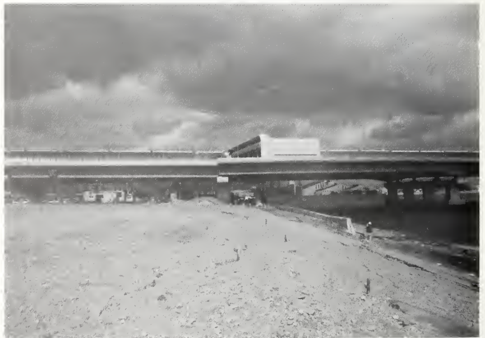
Figure 4.2.42 Distant view of the Shukugawa Bridge showing lateral deformation of the foundation soils and spreading to the right (to the center of the channel).
