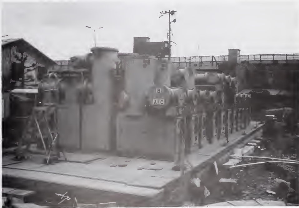
Figure 5.4.65 A 77 kV and 6.6 kV gas insulate distribution substation.
