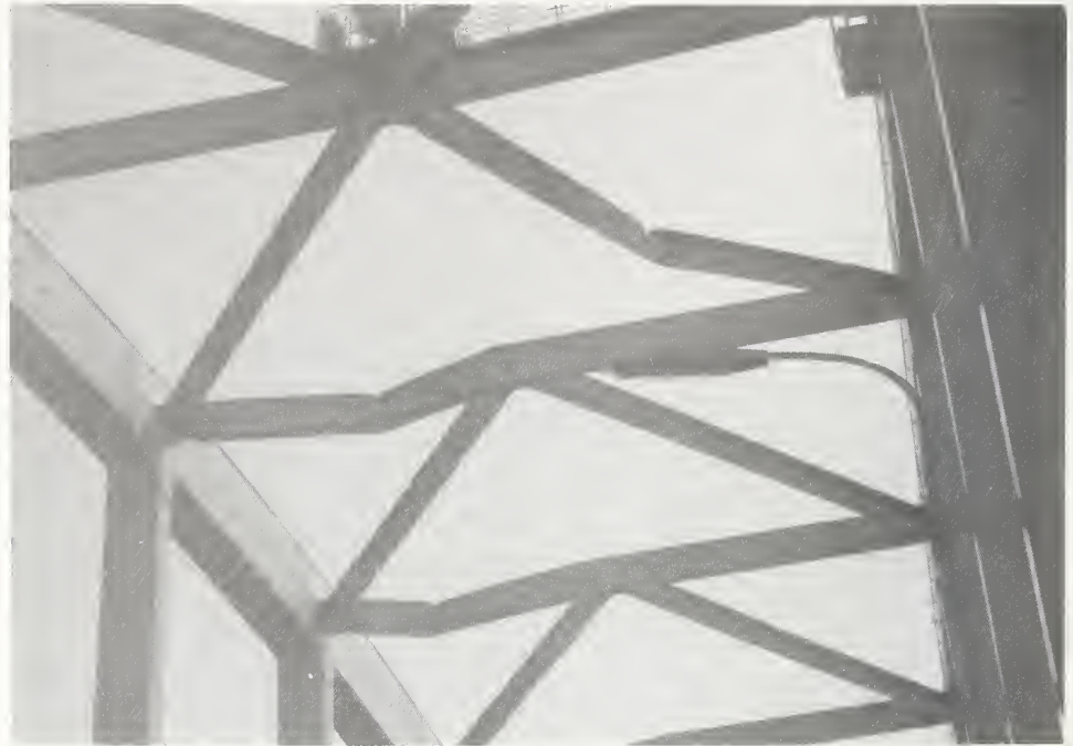
Figure 4.2.8 Buckled cross-members in Upper Chord, Rokko Island Bridge.
