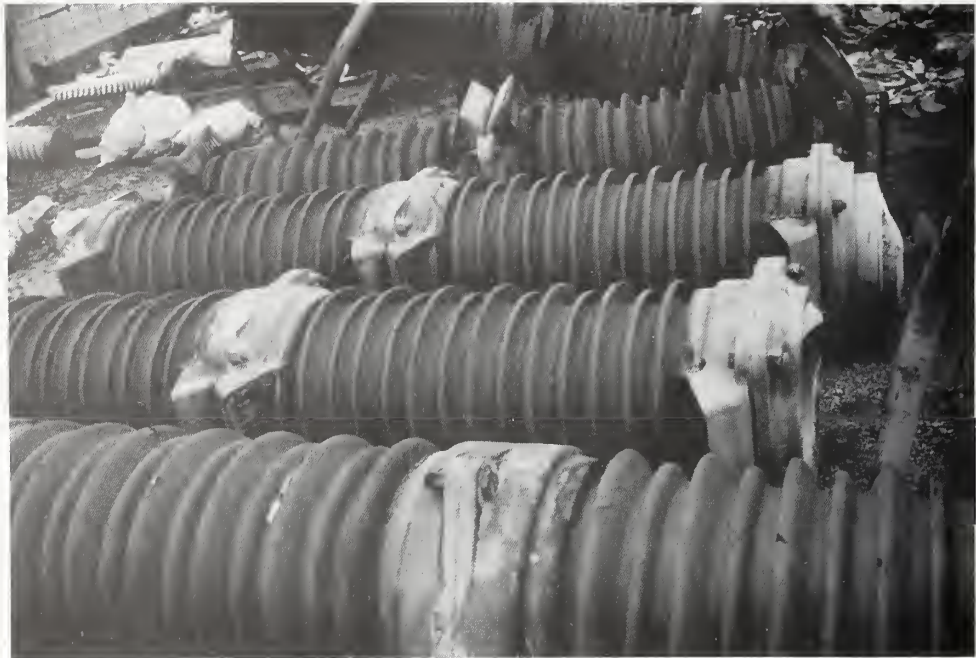
Figure 5.4.31 Damaged 275 kV lightning arrester in the grave yard.
