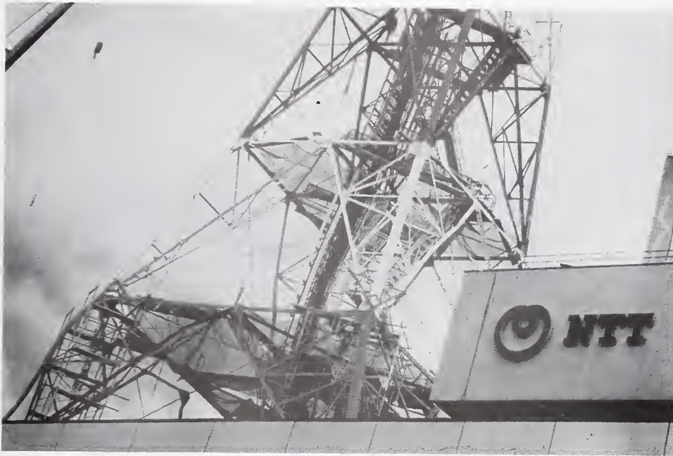
Figure 5.5.1 Microwave tower on top of a central office which was damaged and later removed.
