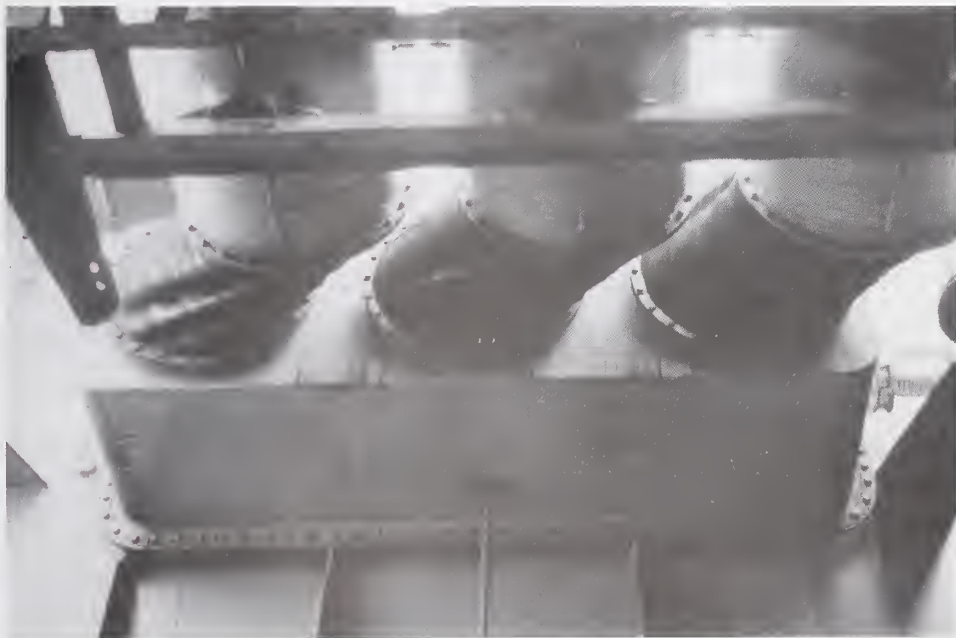
Figure 5.4.34 Offset in bus covers caused by the failure of transformer anchorage and its movement.
