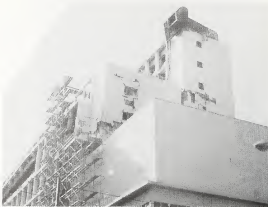
Figure 3.4.23 Collapsed penthouse structure.
