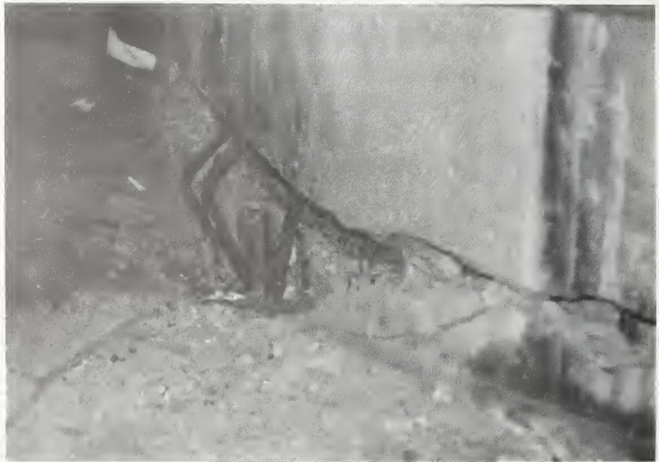
Figure 4.2.12 Failure at top of buried column, Pier P1, Mukogawa Bridge.
