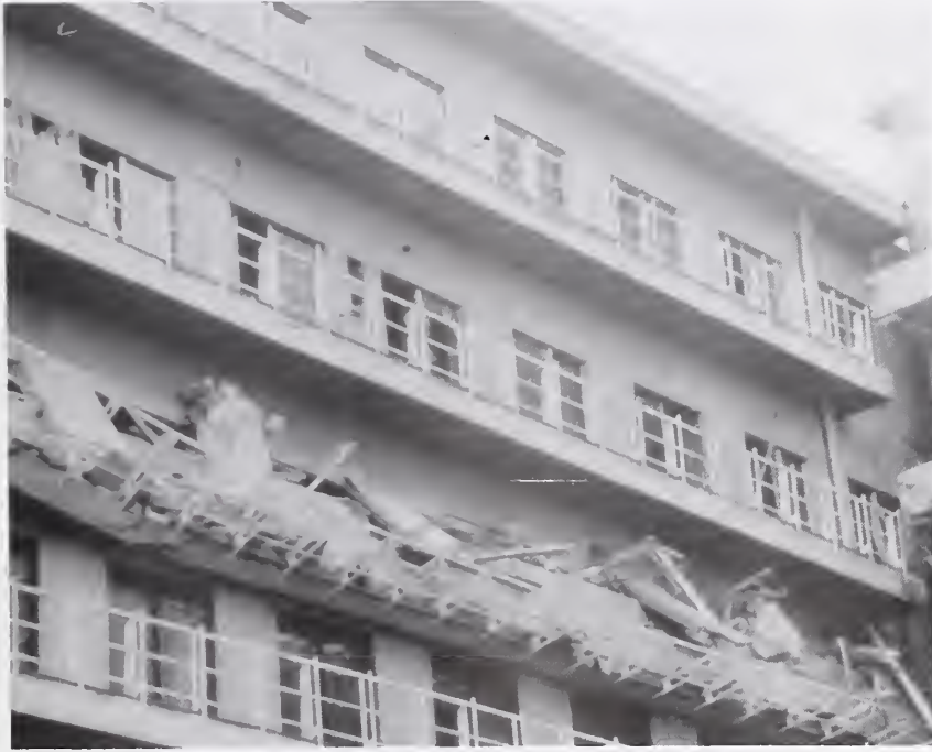
Figure 3.4.25 Collapsed upper story, northeast corner - West Kobe Citizens' Hospital.
