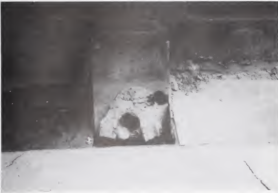
Figure 5.5.11 Settlement of a walkway adjacent to a building shears conduit and cables.
