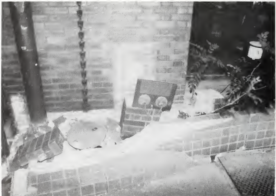
Figure 6.2.12 Standpipe connection severed at street level.
