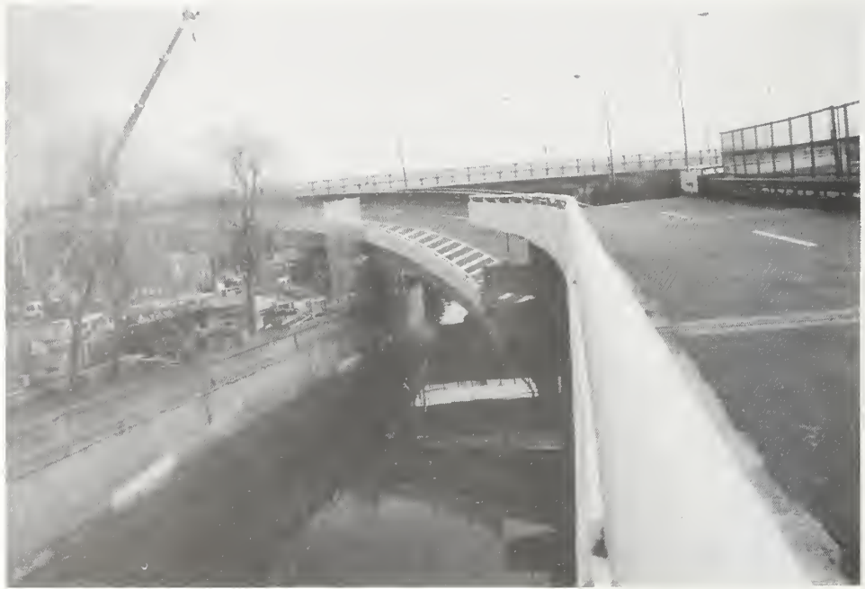
Figure 4.2.28 Collapse of Northeast Ramp at the Minatogawa Interchange.
