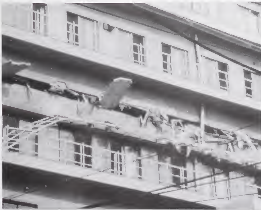
Figure 3.4.26 - Collapsed upper story, northwest corner - West Kobe Citizens' Hospital.
