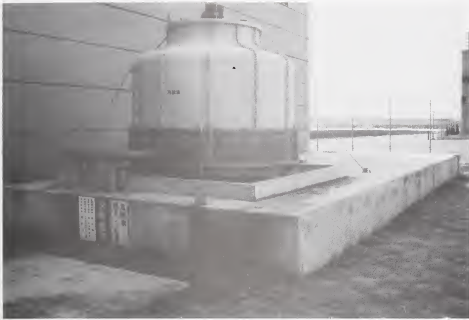
Figure 4.4.22 Cooling tower and water tank for emergency engine-generator.
