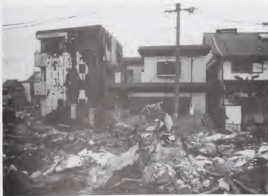
Figure 6.2.18 Burned out structure constructed from fire resistive materials.
