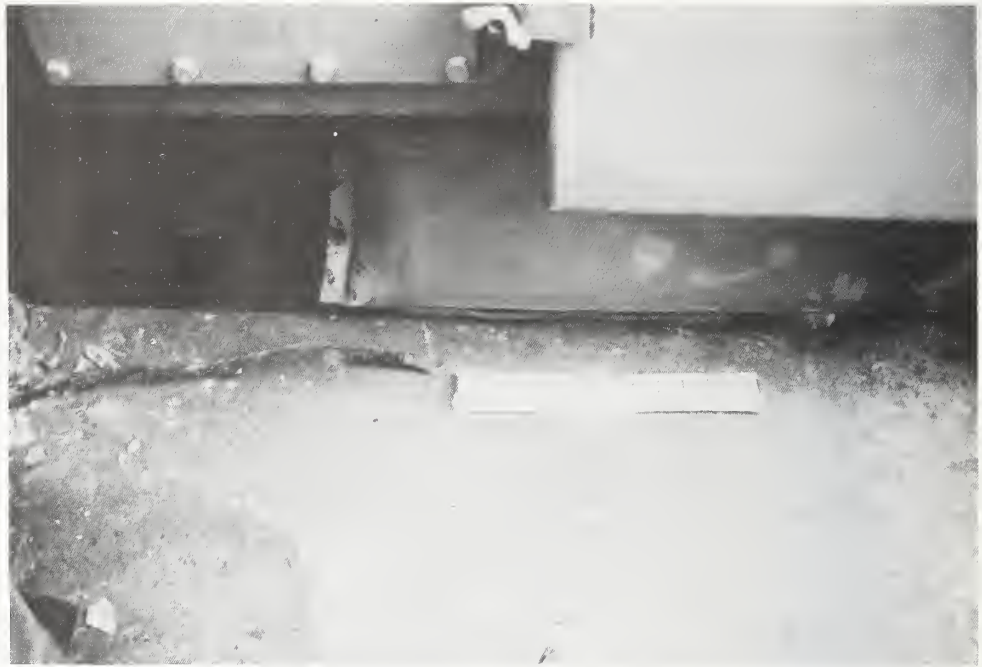
Figure 5.4.35 Transformer control cables were almost sheared off due to movement of the transformer.
