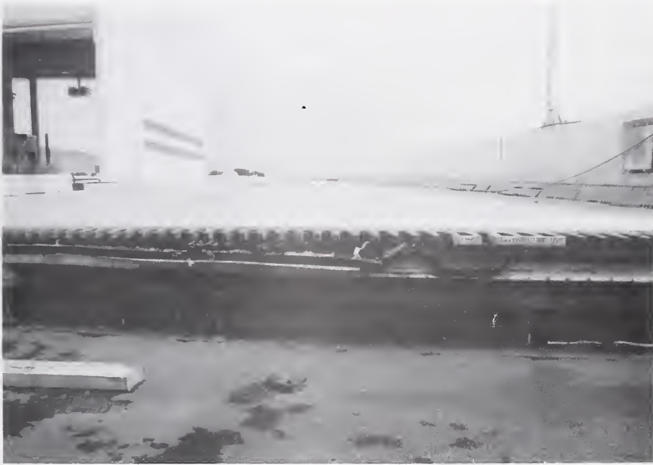
Figure 4.2.43 Vertical offset in the expansion joints above Pier 134 of the Shukugawa Bridge due to bearing failure on the best cap below.
