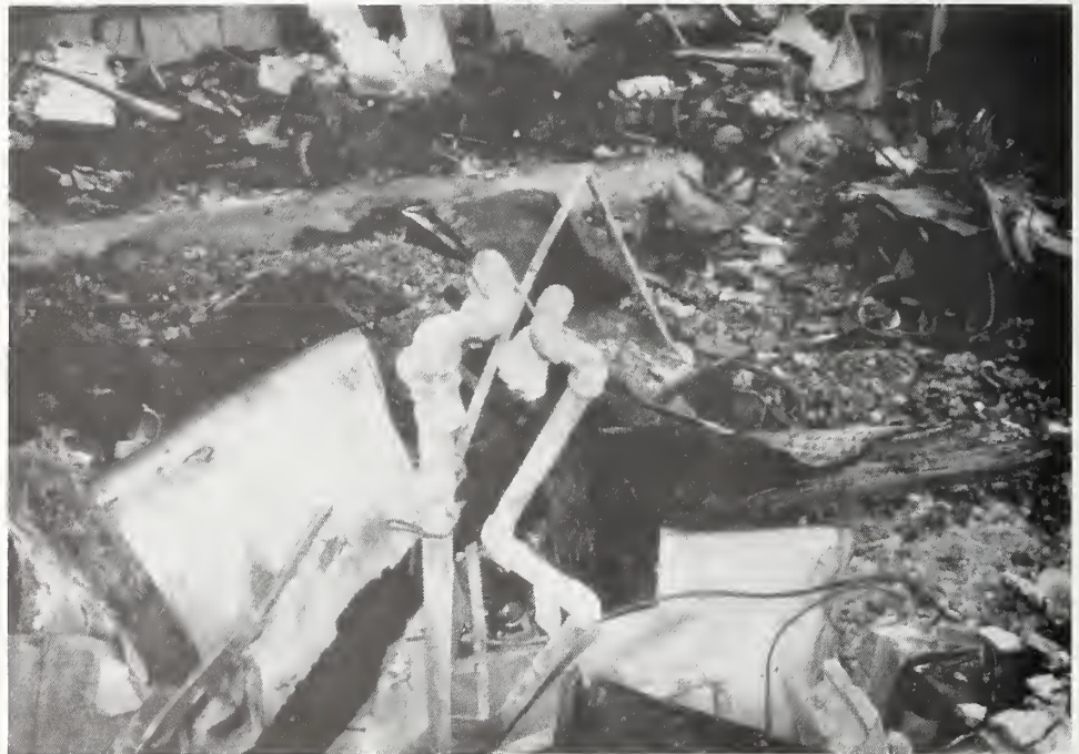
Figure 6.2.4 Broken gas meter connection.
