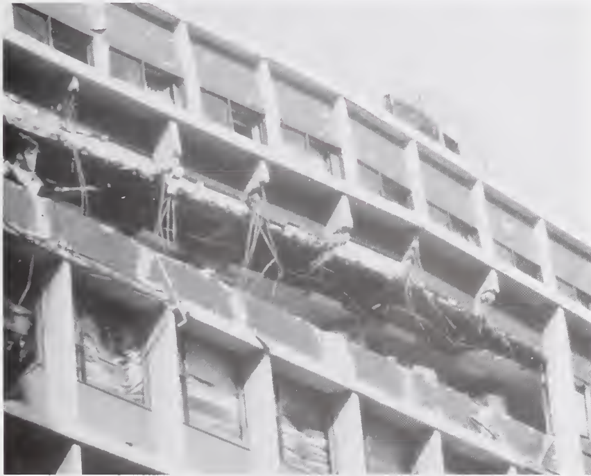
Figure 3.4.22 Upper story collapse - Downtown Kobe.
