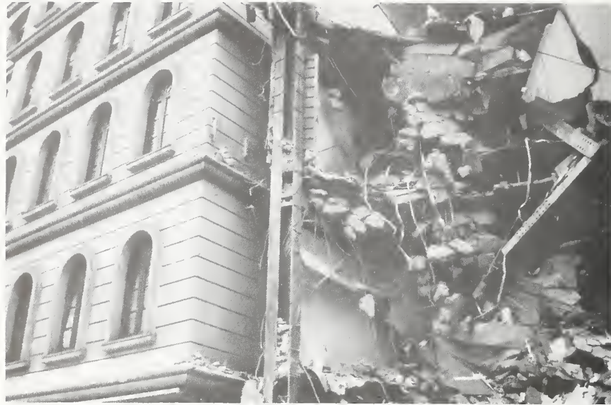
Figure 3.5.22 Collapse of the 3-story Tanigawa building on Flower Road in Kobe. This two-way steel frame was constructed of H-shape beams welded to columns.
