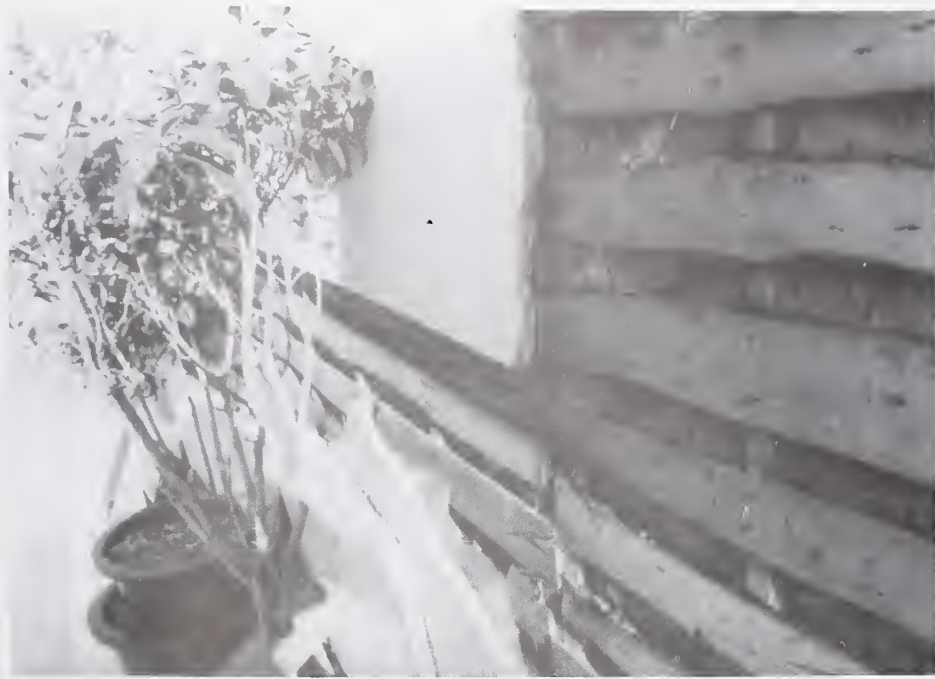
Figure 6.2.13 Example of okabe construction with portions of the fire resistive mortar displaced by the earthquake.
