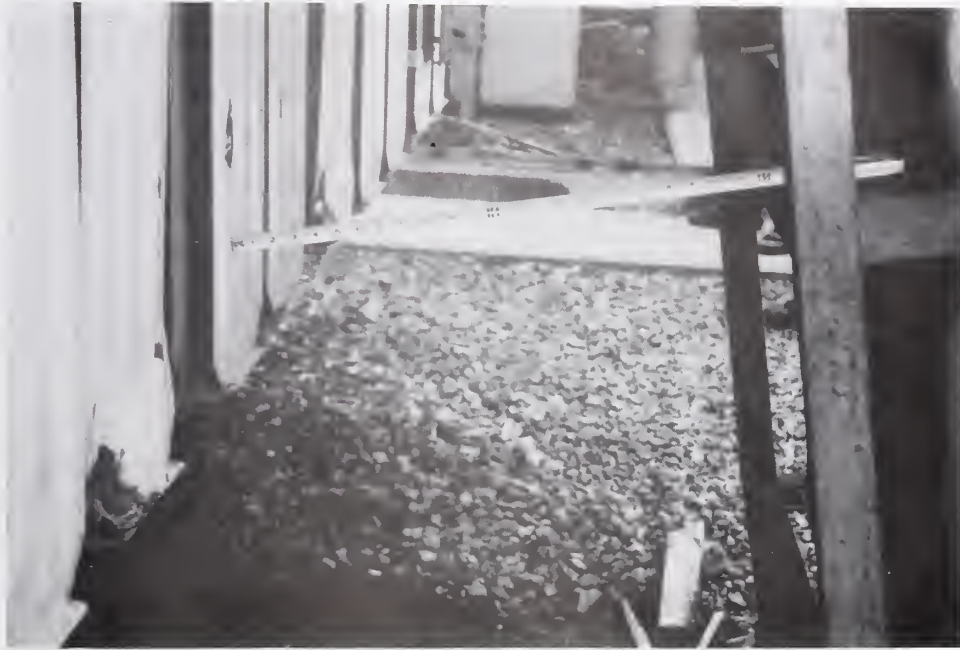
Figure 5.4.64 Movement of the transformer after its anchorage failed allowed the radiators to hit a nearby structural support causing a leak.
