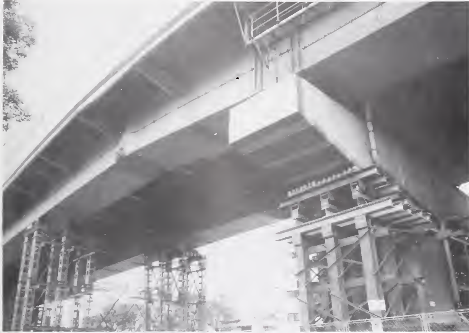
Figure 4.2.20 Compressive failure in lower flange of steel box girder between Piers 238 and 239 of Hanshin Expressway.
