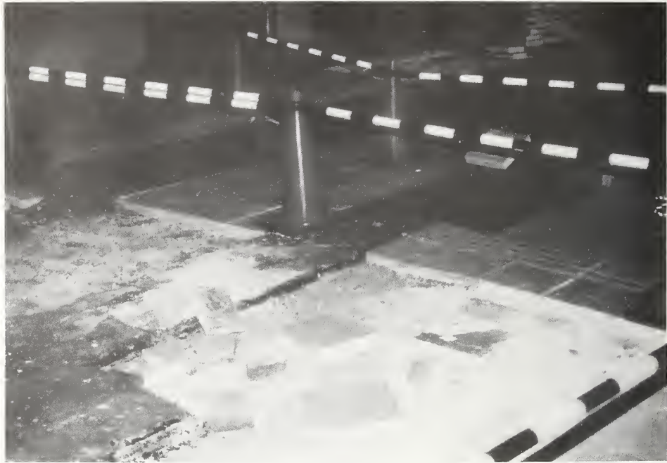
Figure 4.4.26 Subsidence in sidewalk and repaired sidewalk outside the Kansai Terminal Building.
