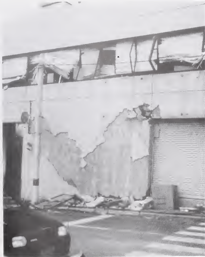
Figure 3.4.17 Second story collapse - Miyagi Hospital.
