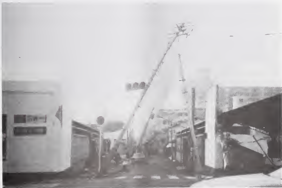
Figure 5.4.69 Some poles failed due to inertial loads or were pulled down by other fallen poles.
