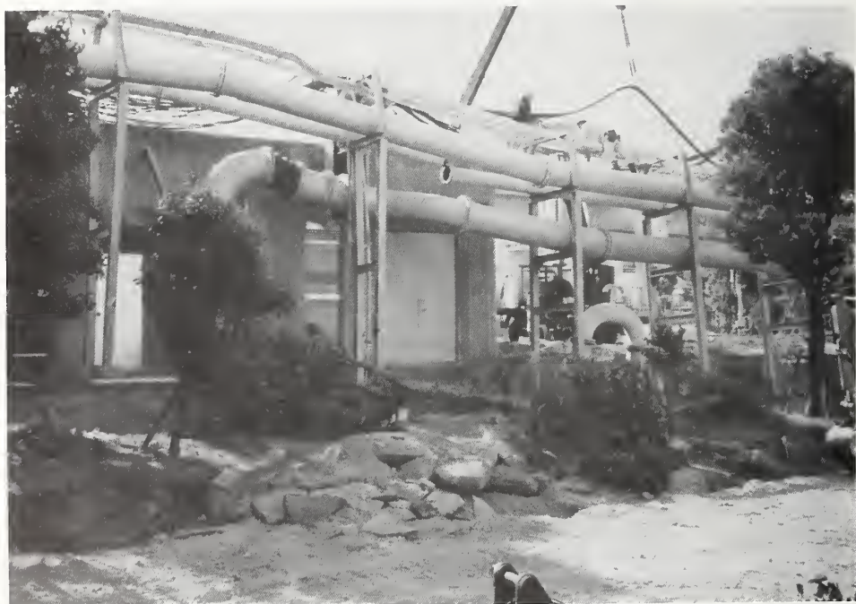
Photo 38 Filter building support pipes failed allowing the building to move and settle differentially.
