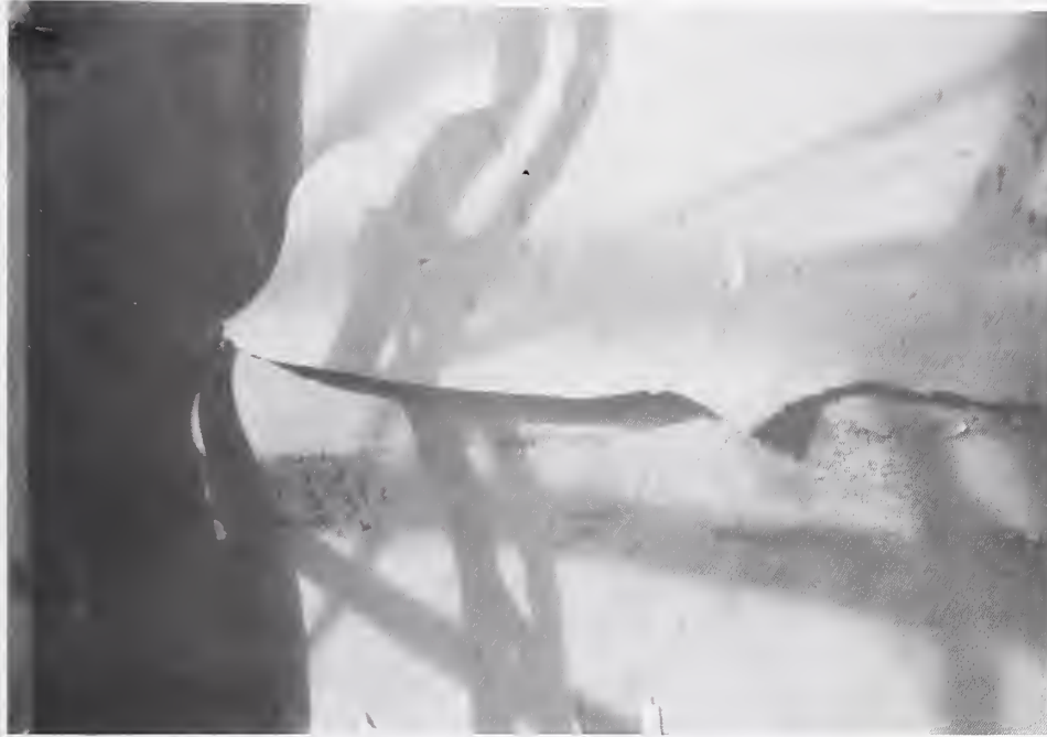
Figure 4.2.37 Fracture at mid-height of Pier 584 of westbound Route 3.
