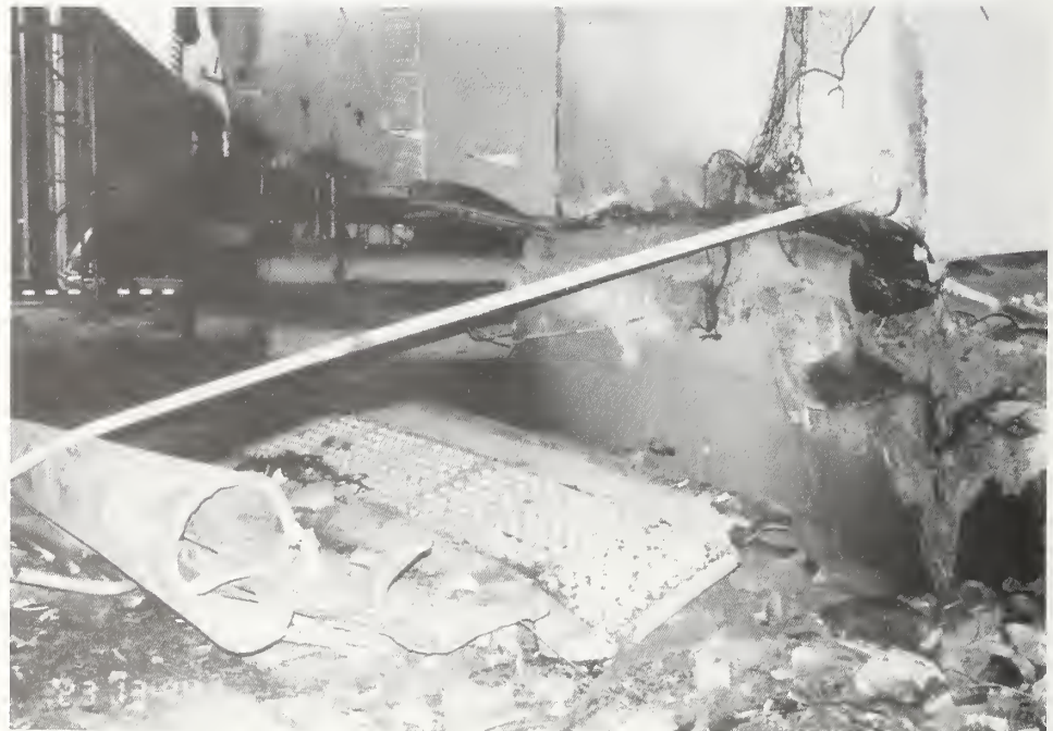
Figure 4.2.34 Pier 55, Route 3 near Tateishi showing buckled steel plate on ground.
