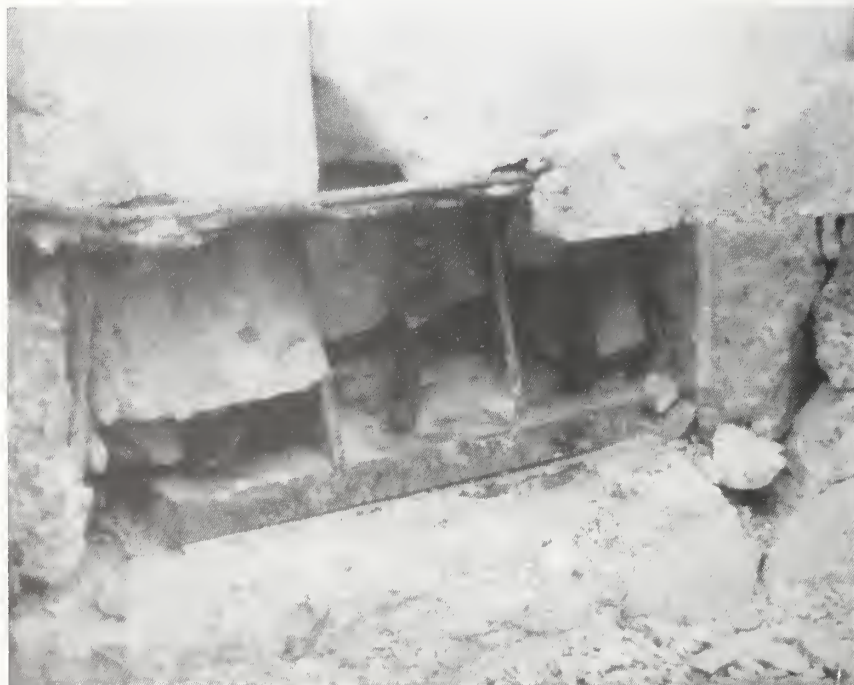
Figure 3.5.36 SAGA Building, anchor bolt was pulled out about 10 cm.
