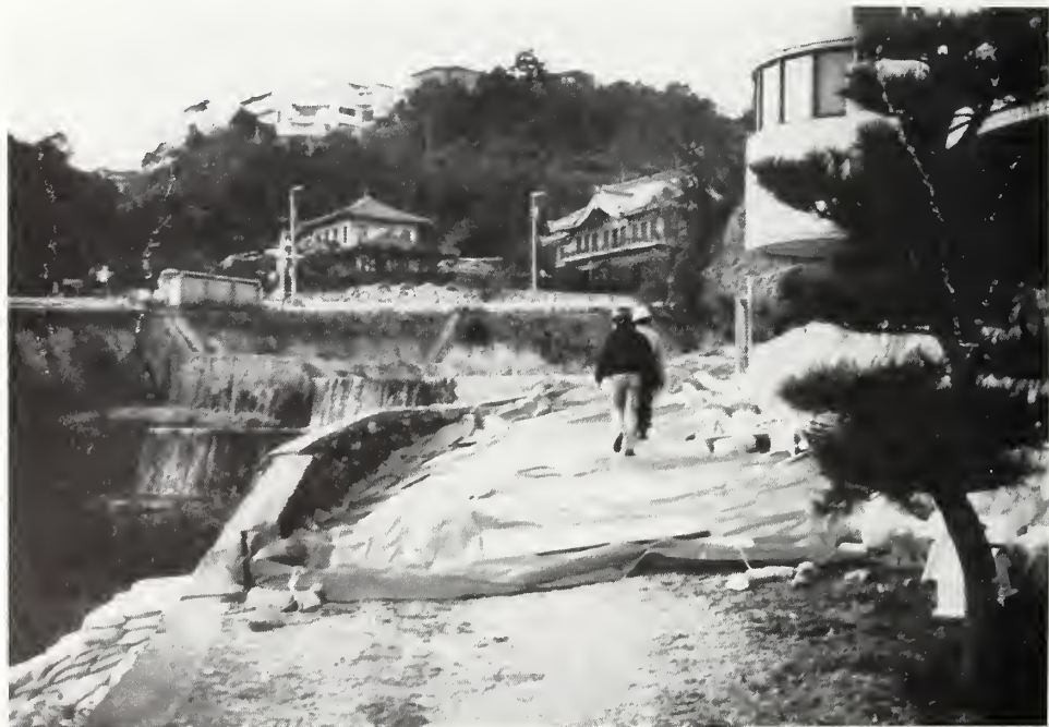
Photo 14 The retaining wall on the left cracked damaging the overflow line from the Motoyama Plant's intake box .
