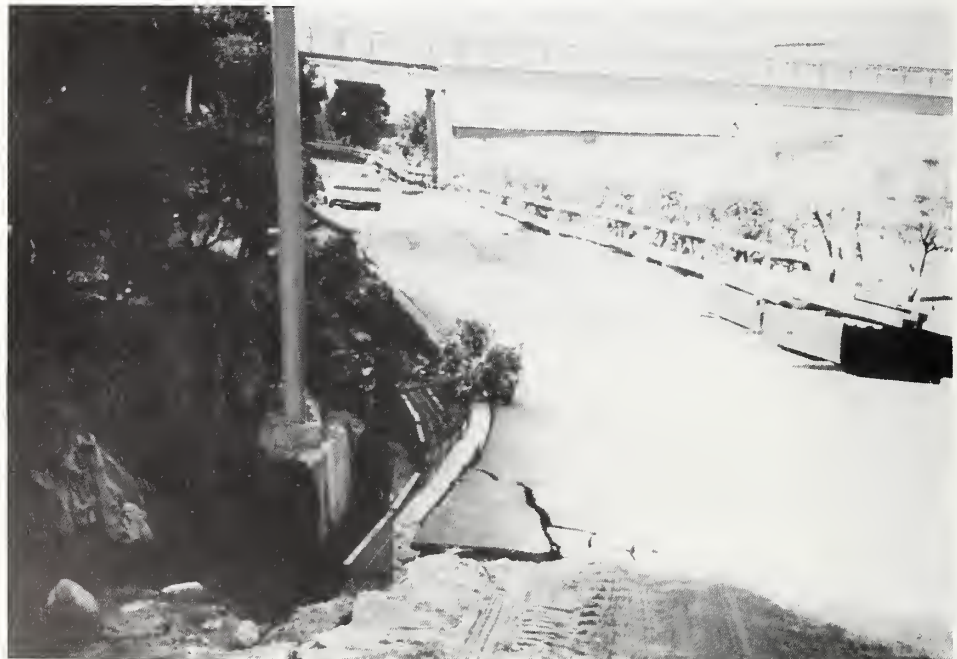
Photo 30 Ground cracking behind the retaining wall (which is off to the left).
