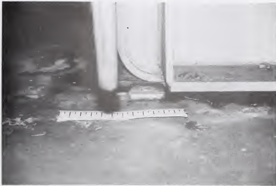
Figure 5.4.33 Bolts anchoring a transformer failed allowing the unit to slide 45 cm and causing damage to bushings.
