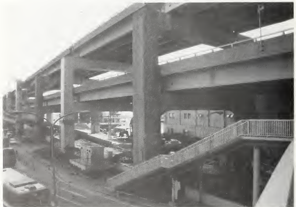
Figure 4.2.25 General view of Kobe-Ohashi Connector near Port Island showing formation of flexural hinges in lower level columns.
