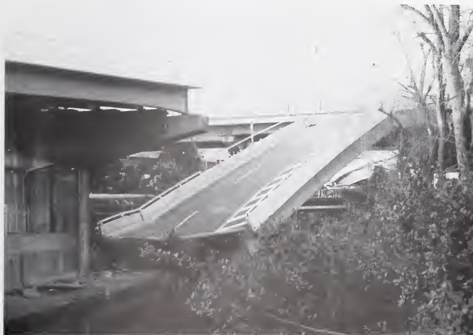
Figure 4.2.27 Collapse of Southeast Ramp at the Minatogawa Interchange.
