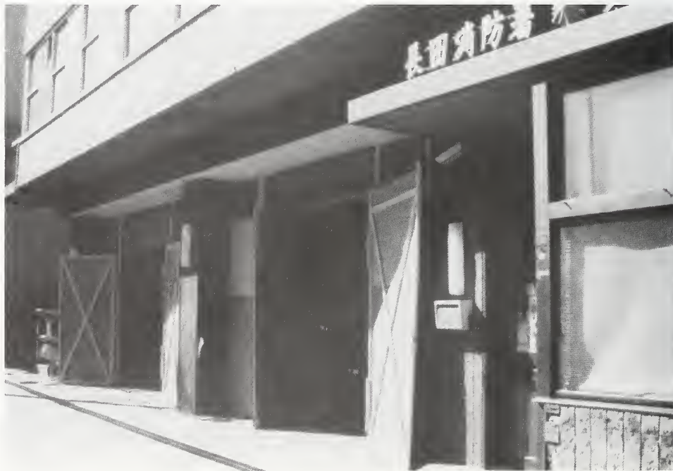
Figure 6.2.28 Fire station damaged by the earthquake.
