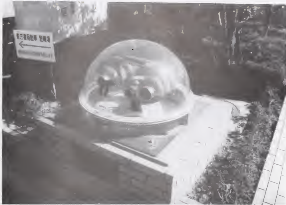
Figure 6.2.21 Seismically reinforced fire fighting water cistern.
