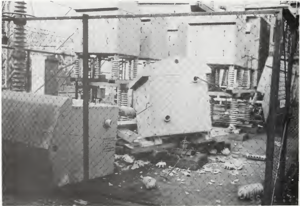
Figure 5.4.58 Neutral resistors failed, a device not used in this configuration in the U.S.
