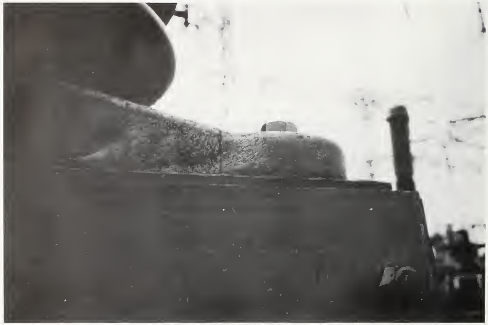
Figure 5.4.22 A cracked cast iron anchor tab on a current-voltage transformer remained in service.
