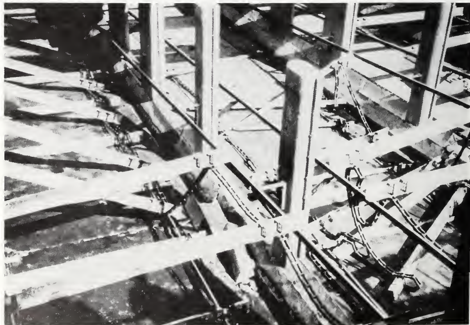
Photo 35 Sludge scraper chain came off sprockets in sedimentation tanks.
