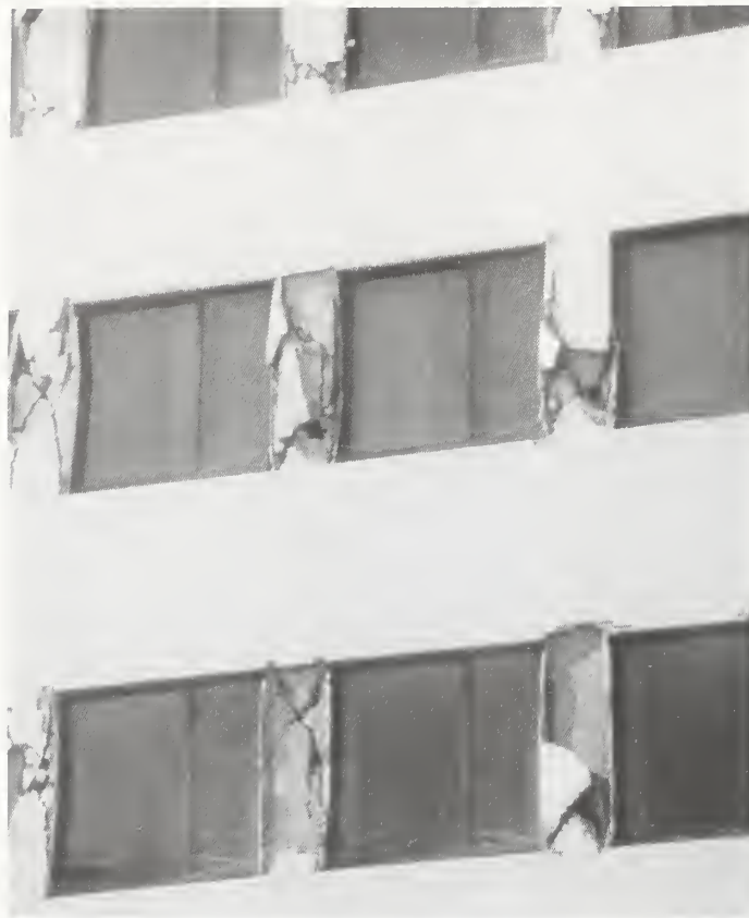
Figure 3.4.10 Short column effects - Otaki Building.
