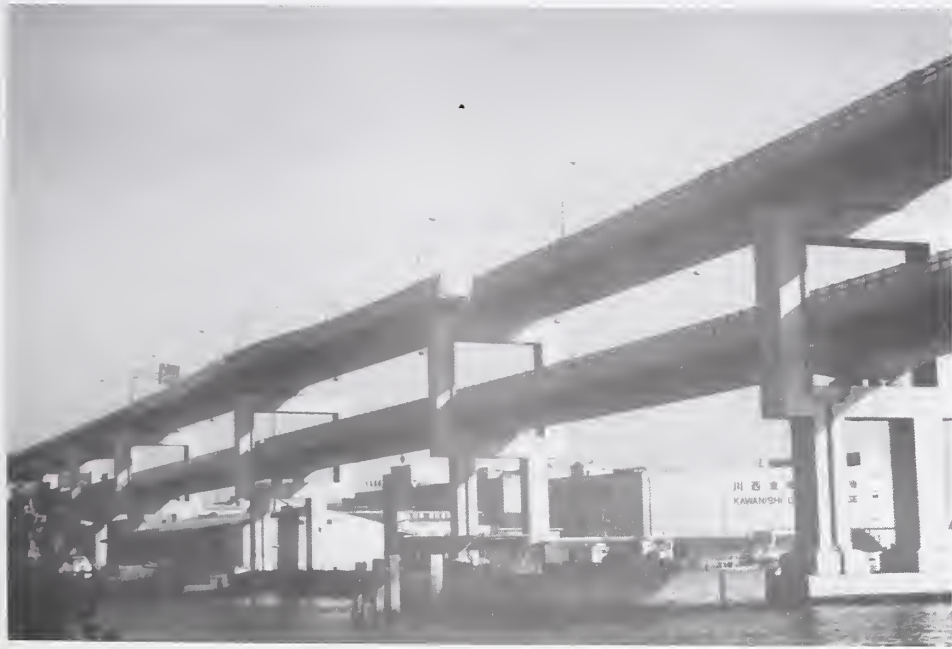
Figure 4.2.13 Lateral offset at Pier 36 in upper level of Hamate By-Pass due to bearing failures at Piers 34 through 38.
