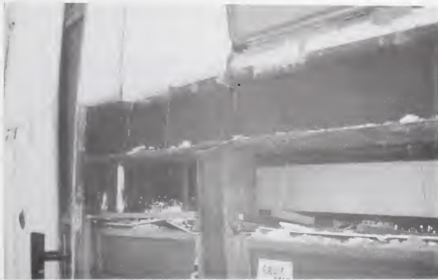
Figure 3.5.20 First floor column to second story column joint fillet weld failure on the east side of the Nairo Hiro Building, downtown Kobe.
