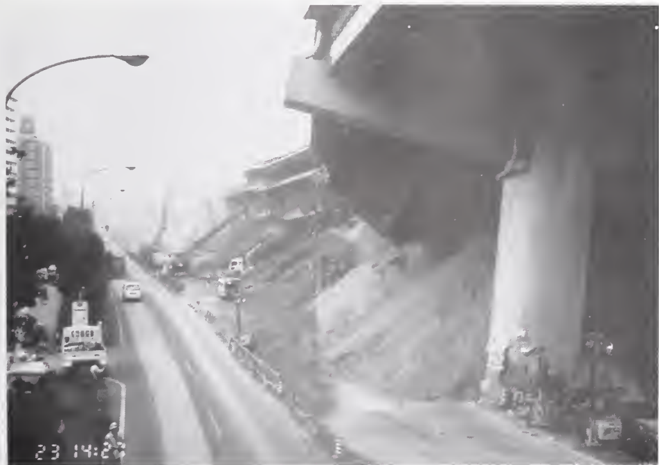
Figure 4.2.14 View of the collapsed Higashi-Nada Viaduct looking west from Pier 125.
