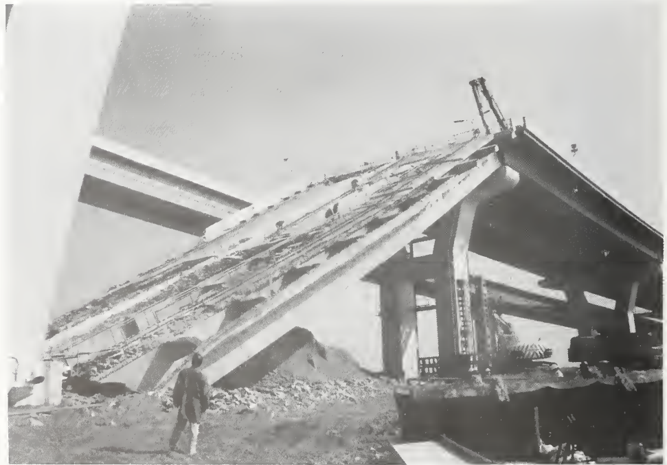
Figure 4.2.2b Collapsed approach span between Piers 111 and 112, Nishinomiya-ko Bridge.
