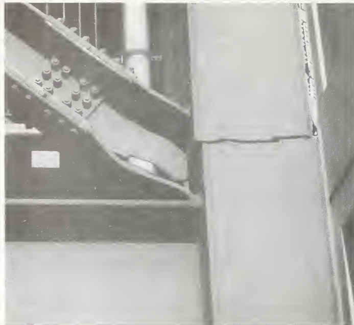
Figure 3.5.41 Complete fracture through a steel column section.
