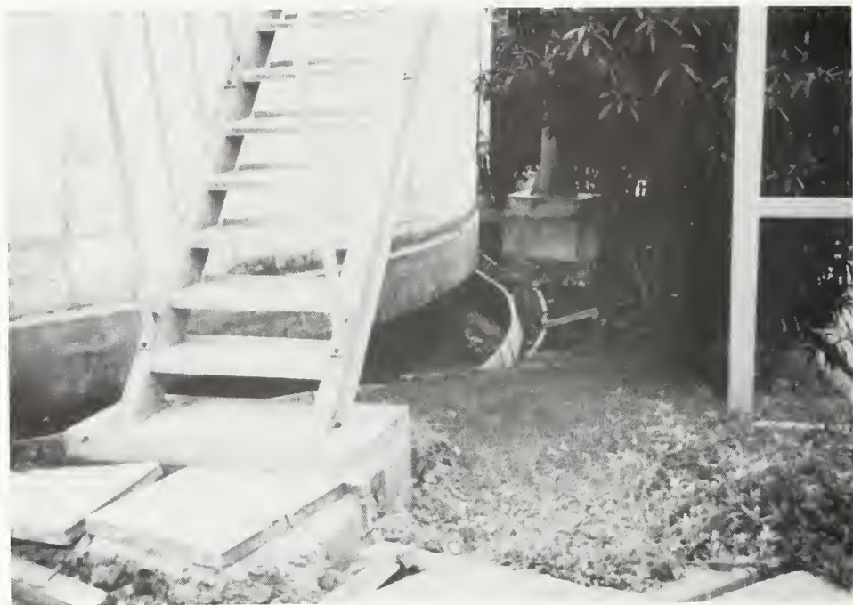
Photo 37 Differential settlement between pipe and non-pile supported structures damaged piping throughout the plant.
