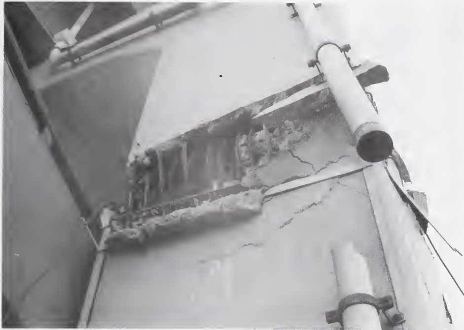
Figure 4.2.26 Hinge formation in east column of Pier 23, Kobe-Ohashi.
