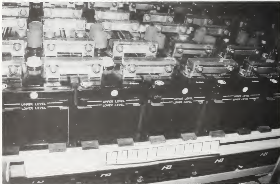
Figure 5.4.41 A different approach using rubber spacers in Japan to restraining cells to battery racks.
