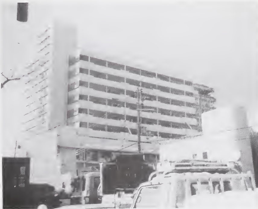
Figure 3.4.18 Fourth story collapse in apartment building.
