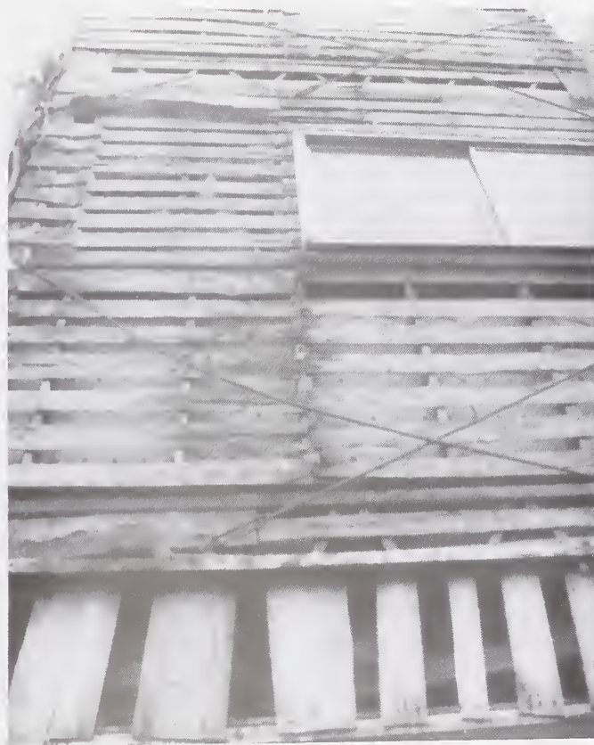
Figure 6.2.14 Example of a structure with mortar exterior after earthquake.
