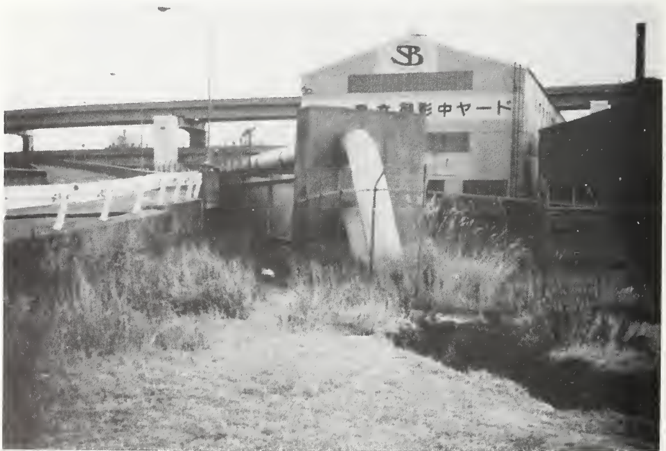
Photo 17 Ground cracking from lateral spread in fill area along a water way. Immediately behind the crack, a pipeline emerges out of the ground to be supported on the bridge.
