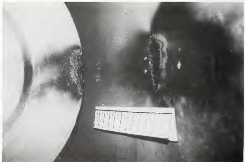
Figure 5.4.36 Movement of transformer damaged cabinet and shorted transformer case the tertiary output.
