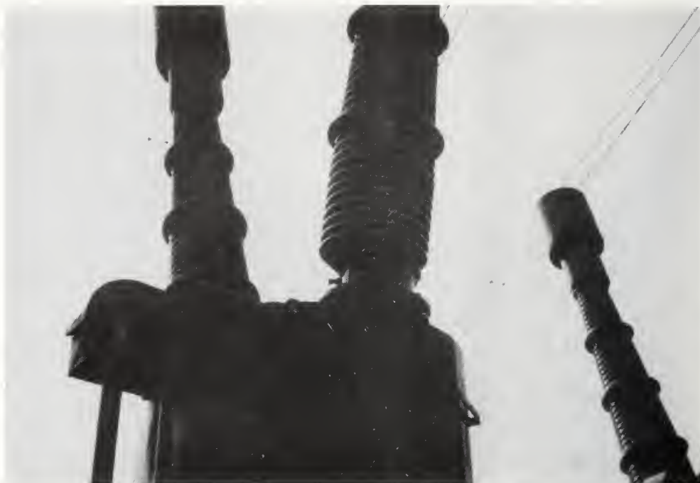
Figure 5.4.25 The porcelain slipped on its lower flange on a 275 kV bulk-oil Circuit breaker.
