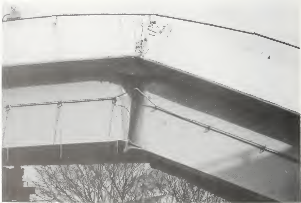
Figure 4.2.29 Girder web failure due to unseating of the Southeast Ramp at Minatogawa Interchange.
