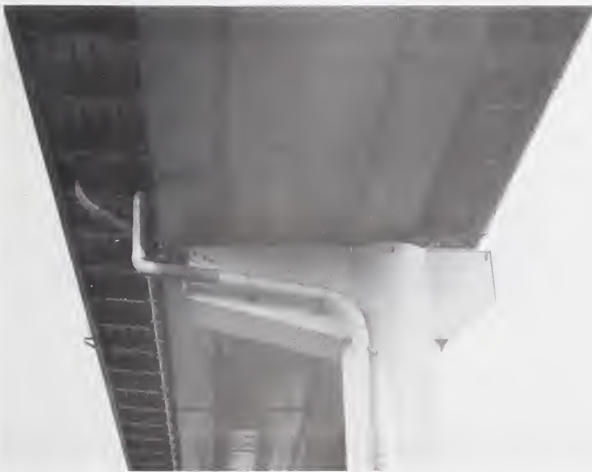
Figure 4.2.38 Failed bearings and lateral offset at top of Pier 586 of westbound Route 3.
