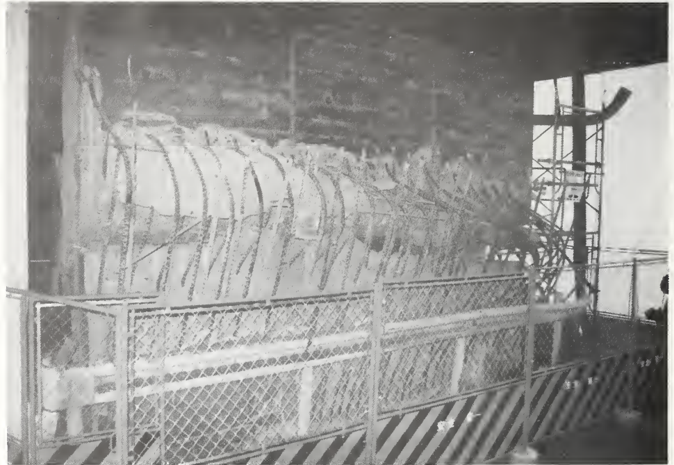
Figure 4.2.24 Shear failure in wall pier (east face), Moribe Viaduct.
