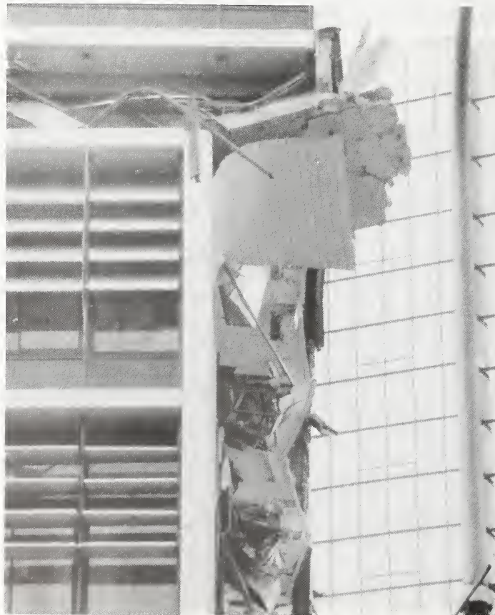
Figure 3.4.24 Collapsed upper story, north end - Kobe City Hall Annex.
