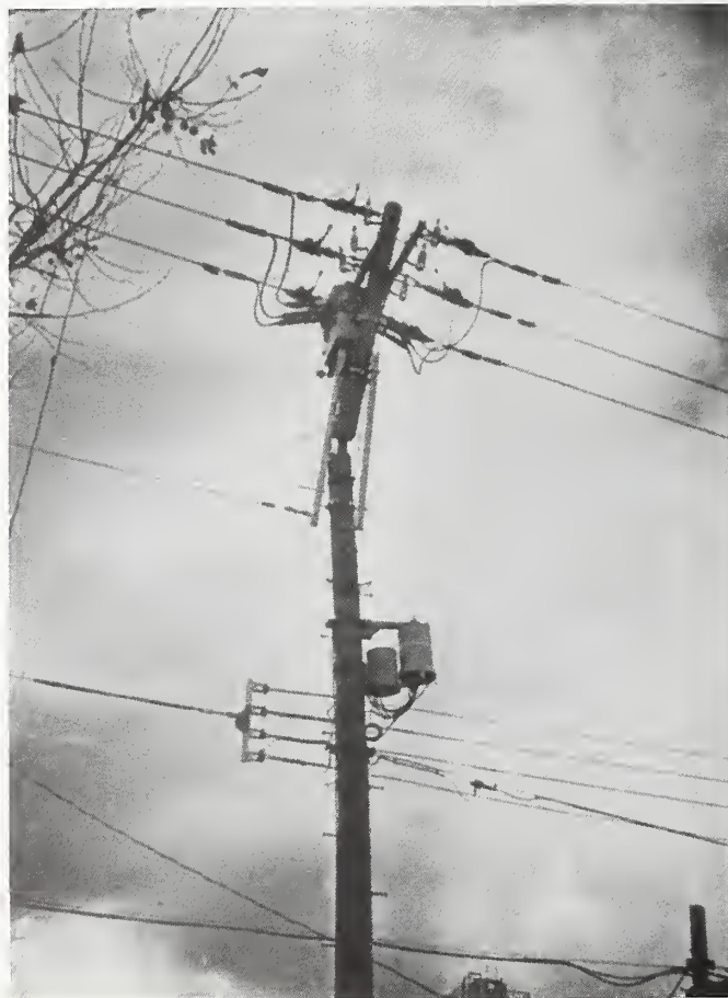
Figure 5.4.67 Damage to the aerial distribution system was severe in many regions.
