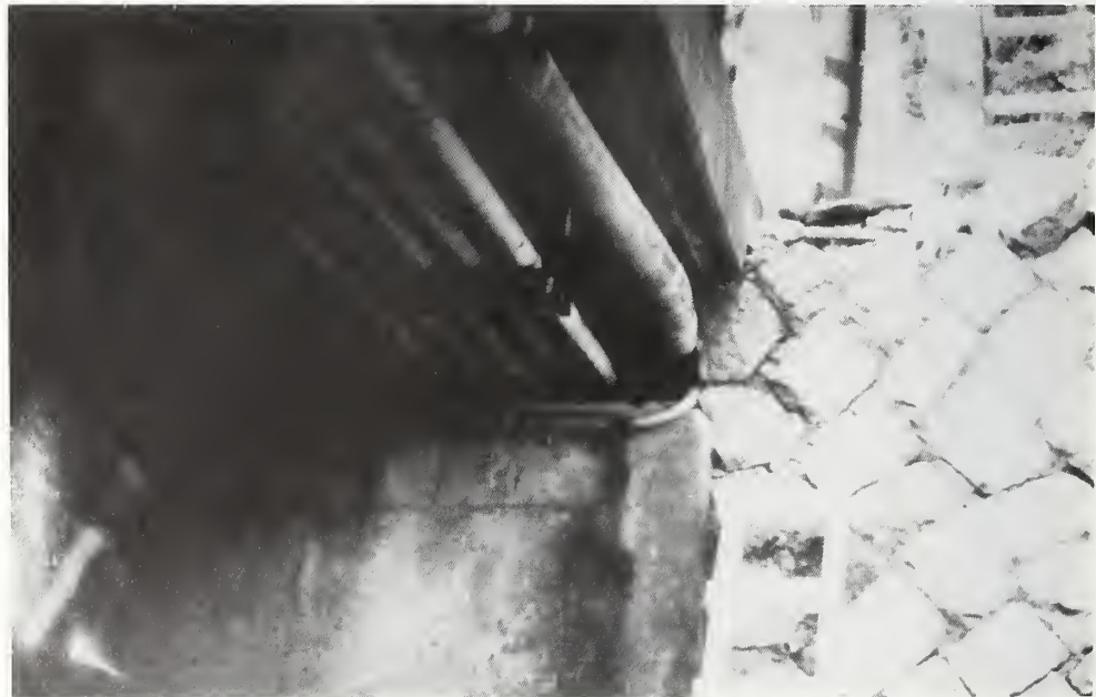
Figure 5.5.9 Conduits carried on bridges were damaged when bridge deck moved.
