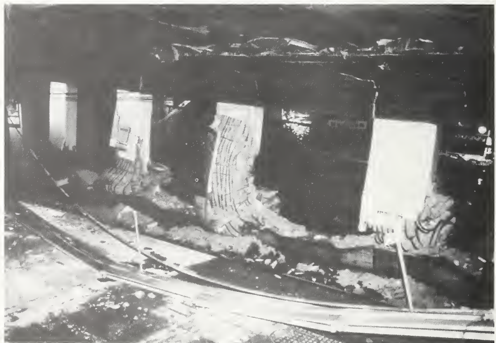
Figure 4.3.20 Compressive failure of center columns at Daikai Station.
