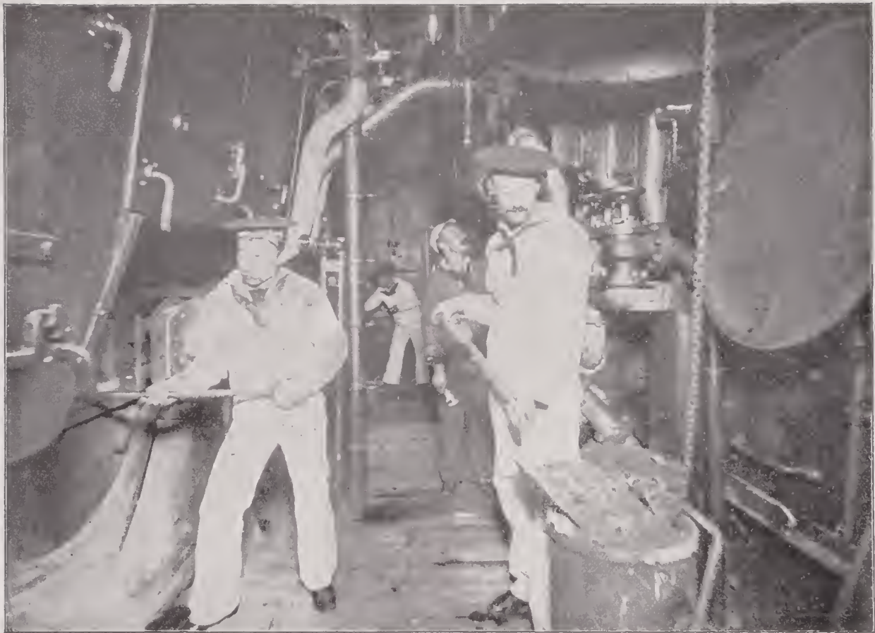
FIRE ROOM OF A UNITED STATES MONITOR —There is probably no more trying situation aboard ship than duty in the fire room. The heat is always very severe, even in the best ventilated ships of the navy, and it is seldom that the men on duty can wear any covering on the upper part of their bodies.
