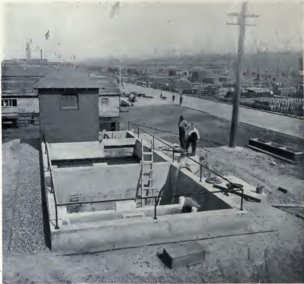
CHLORINATOR HOUSE AT SEWAGE DISPOSAL WORKS INSTALLED FOR EMERGENCY FLEET CORPORATION AT HOG ISLAND SHIPYARD
