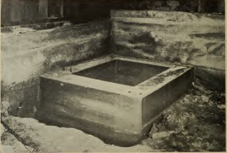
Fig. F—Concrete work completed and ready for the attachment of the cover. (Photo by Prof. H. W. Riley).
