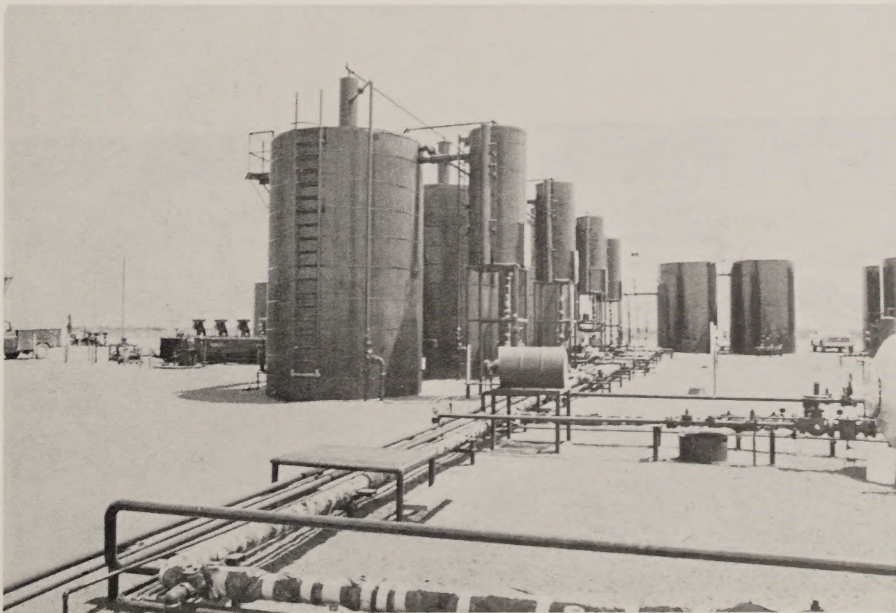
PHOTO 6 - Oil storage facilities at Uvalde.
