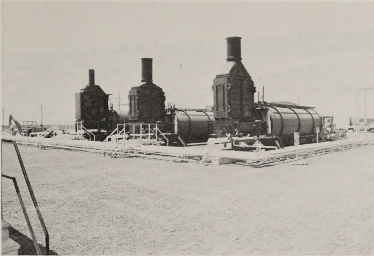
PHOTO 5 - Oil-fired boilers utilized to produce the steam needed for injection into the tar sands deposit at Uvalde facility.
