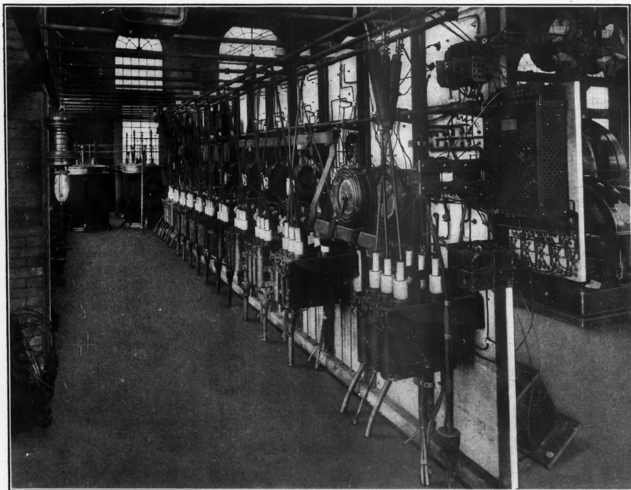
REAR VIEW OF SWITCHBOARD, YORK RUN POWER PLANT, H. C. FRICK COKE COMPANY
