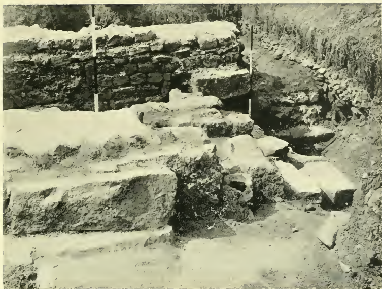
Fig. 31. North-west gateway: south-west guardroom B from the north-east, with roadway in foreground, two pivot stones, and (on right) steps.
