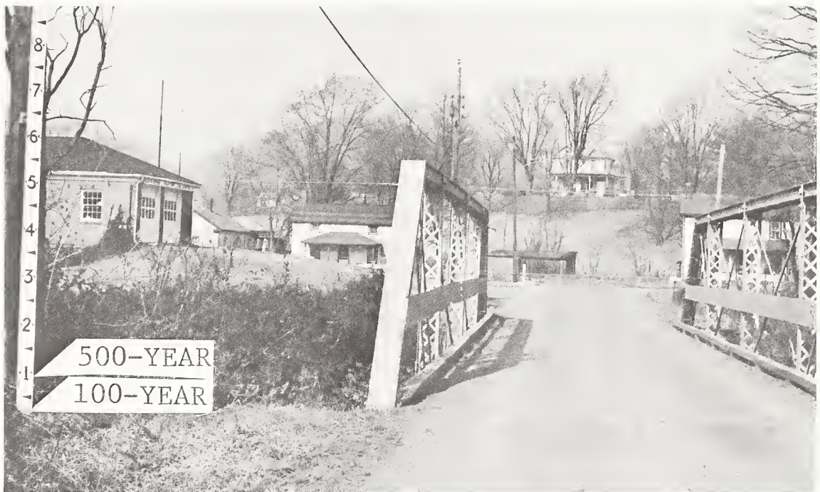
Figure 3. Potential flood stages at State Route 601 crossing of Little Calpasture River at Augusta Springs.
