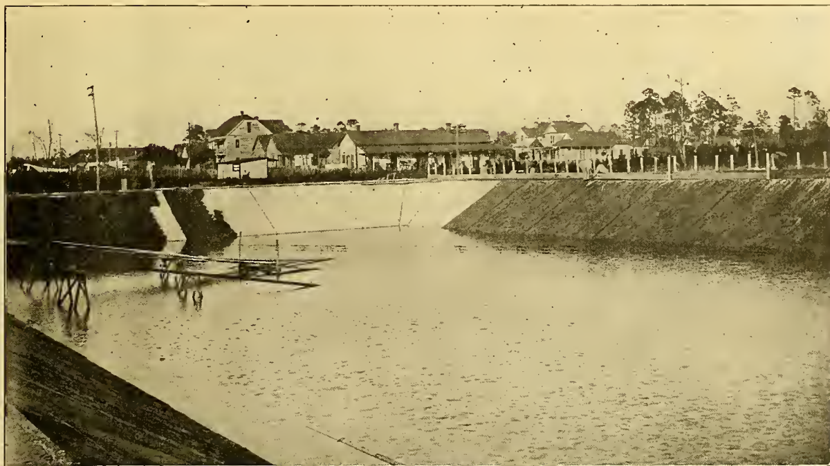
THE CITY'S NEW RESERVOIR IN COURSE OF CONSTRUCTION. When completed will hold one million gallons of water.
