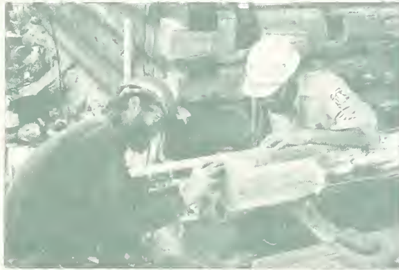
Sourdough Lookout Restoration Project: Warren Miller (left) and Ali Abusaidi. Photo by Cindy Schacher
