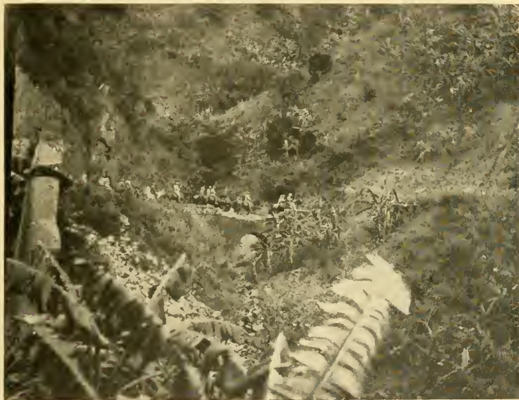
A CULVERT OF THE MILITARY ROAD PARTIALLY DESTROYED BY THE SPANIARDS
