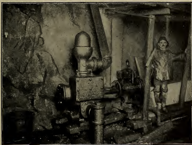
Photograph taken in Pennsylvania and Long Island R. R. Tunnel. Cameron Station Pump handling the drainage water, which seeps through the rock and earth that separate the tunnel from the river bottom.
