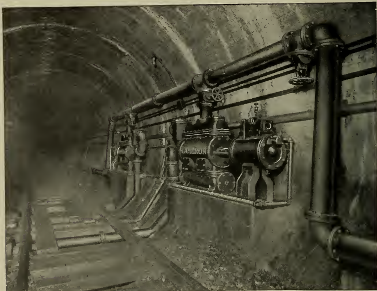
Cameron Pump for Drainage in Harlem River Tunnel, New York Subway.
