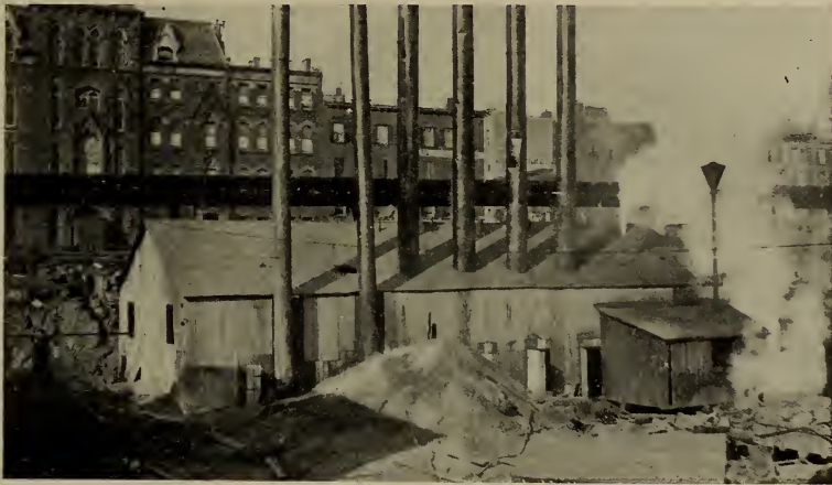
FIG. 1.—Temporary Power House, Pennsylvania Terminal.
