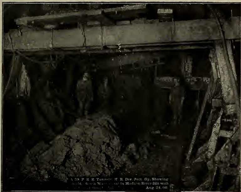
Interior of Shield in P.R.R. North River Tunnel, Showing Silt Entering Through One Open Door.
