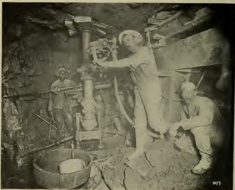
Ingersoll-Rand Rock Drills in Heading of One of the East River Subway Tunnels.
