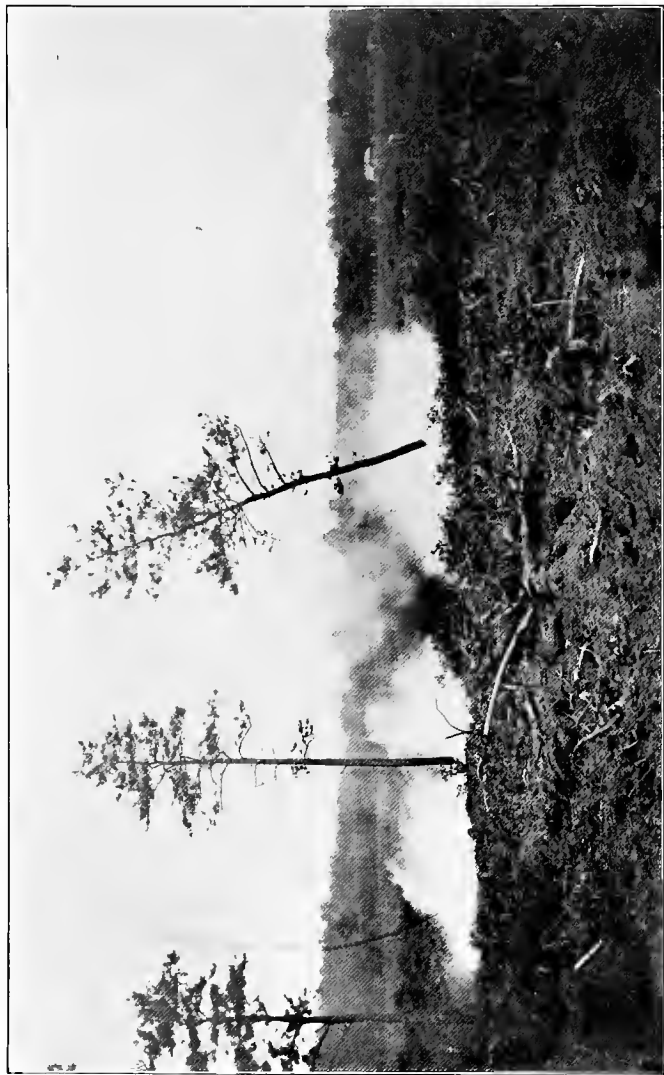
Rooting up trees with dynamite. Taken on Long Island. The dynamiter and his helper can blow up 157 stumps, from four to six feet in diameter, in a day, while two men by old-fashioned methods could remove but two.
