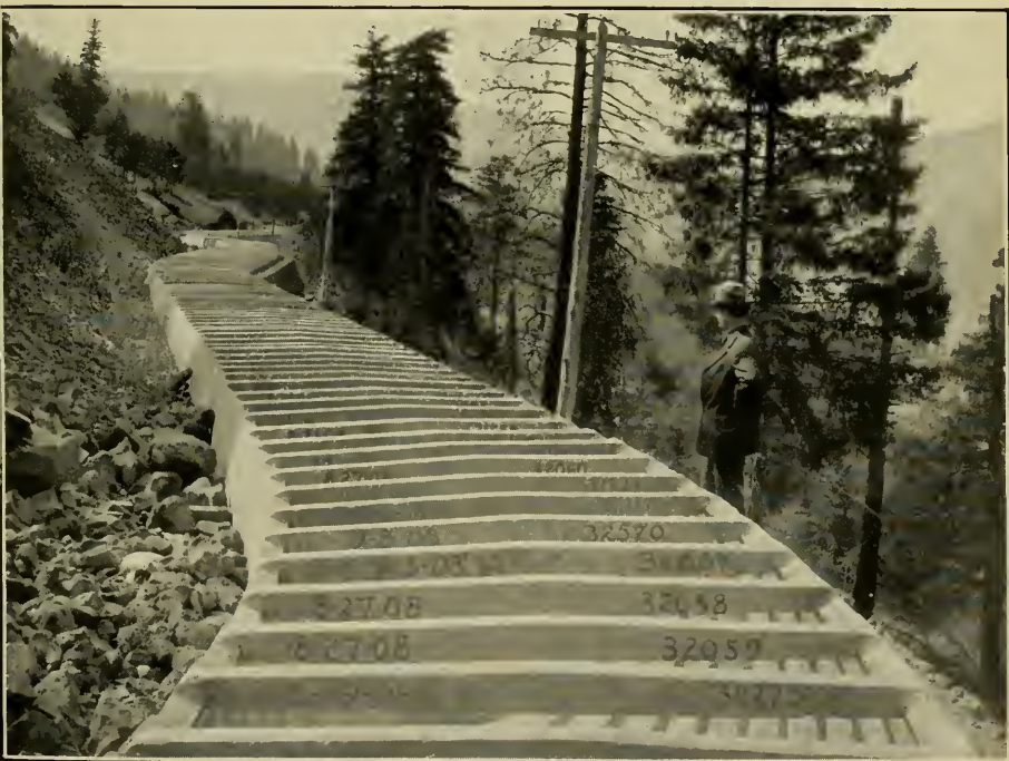
2. CONCRETE FLUME BUILT IN SHORT SECTIONS FOR MAIN TIETON CANAL, YAKIMA PROJECT, WASHINGTON.
