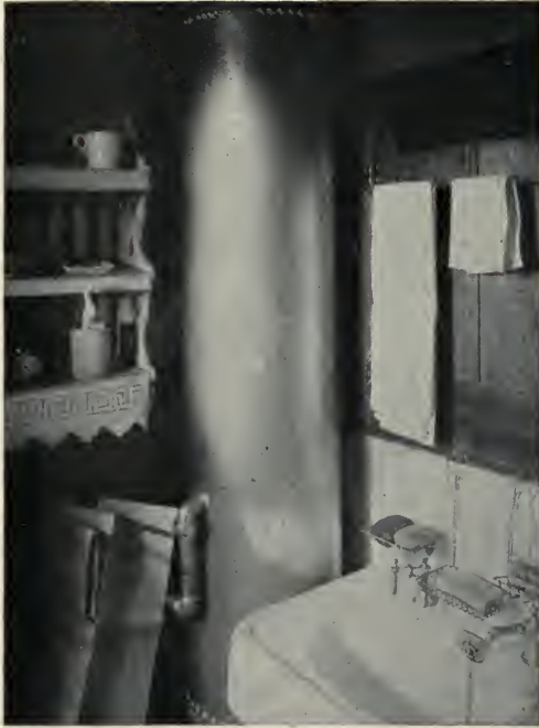
The kitchen boiler in this little bungalow was placed on the other side of the kitchen partition, bringing it into the bathroom, which room it serves to heat
