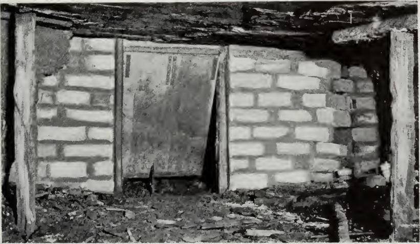
FIG. 47. Explosion-door in concrete-block stopping in District V
