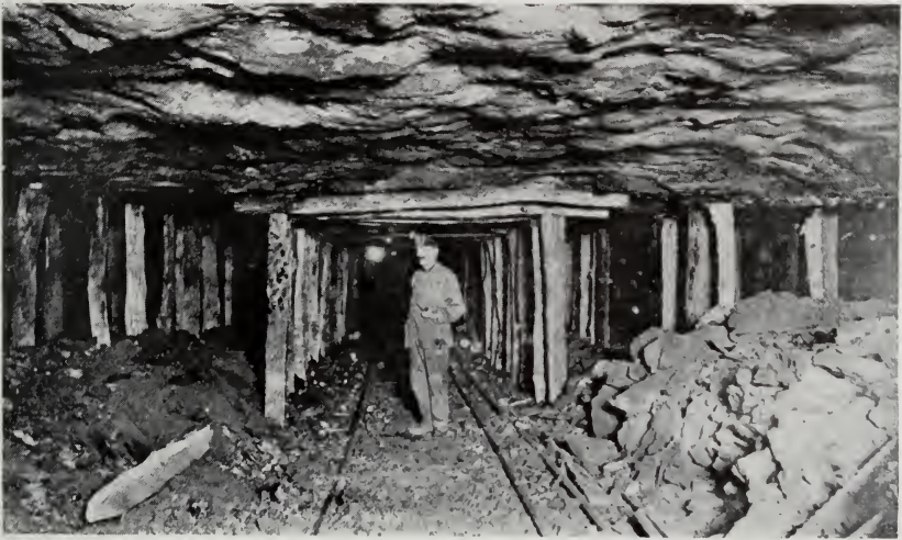
FIG. 43. Alternation of good and bad roof
