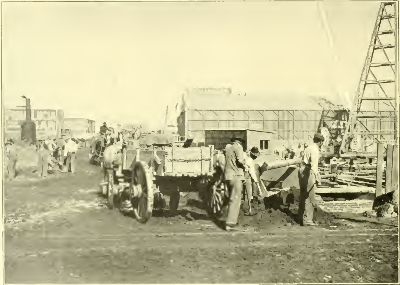
Rebuilding San Francisco—Laying Foundation for Fireproof Building at California and Market Streets.
