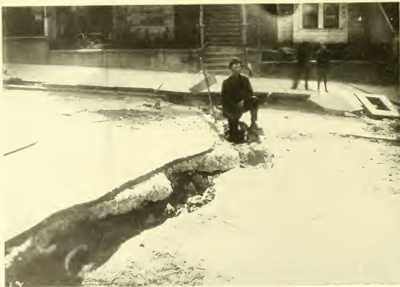
The Break in the Street on Van Ness Avenue, near Vallejo Street, caused by Earthquake. Water Mains broken here.
