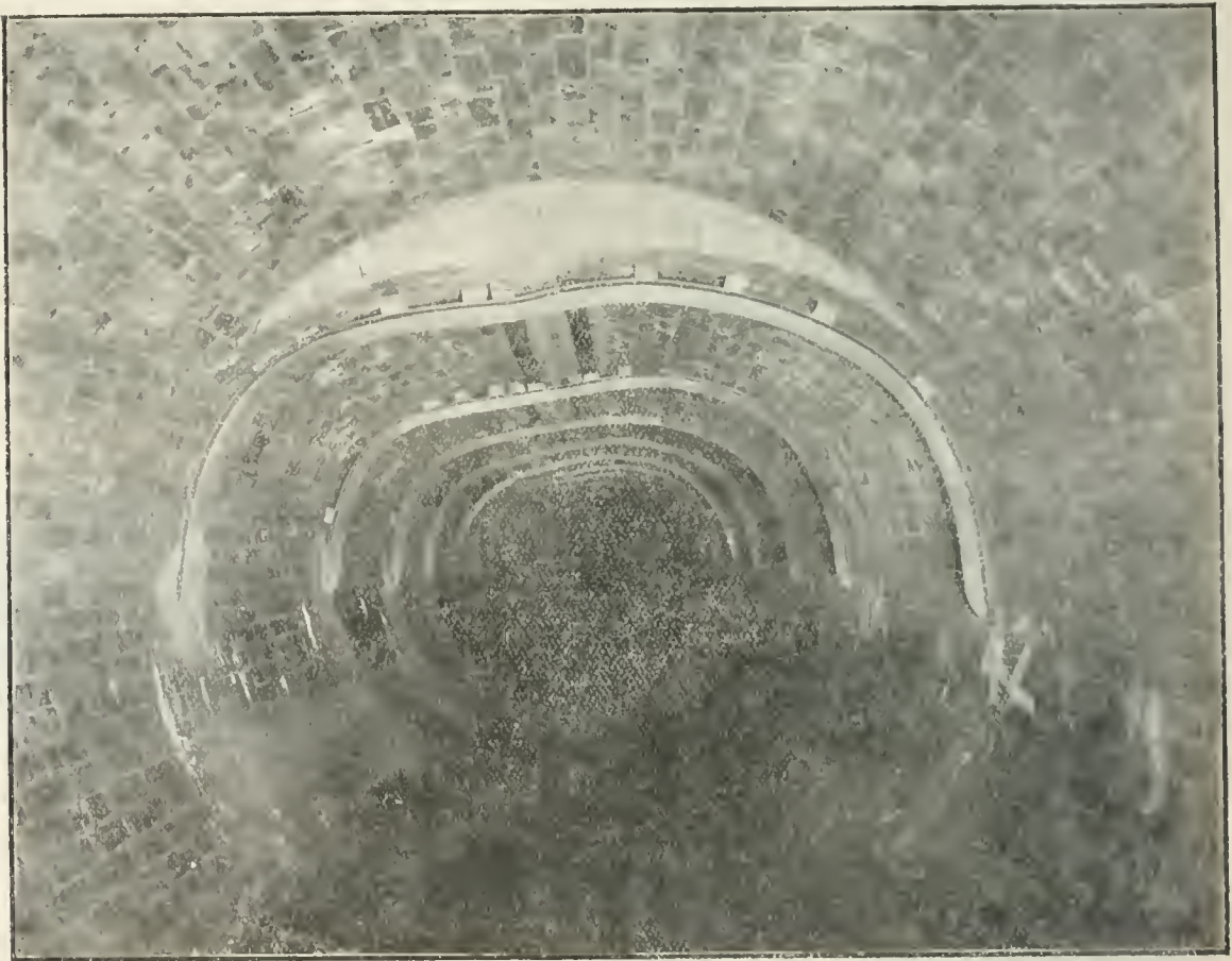
VIEW OF INTERIOR OF DEFECTIVE SEWER (FIG. C).
