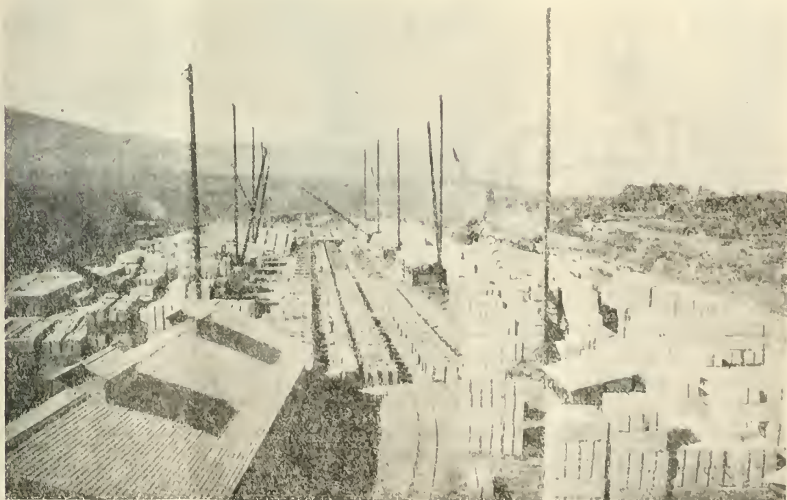
FIG. 9.—OLIVE BRIDGE DAM: BLOCK YARD AND CEMENT STORAGE FROM CONCRETE PLANT. (Tracks at right lead to Sand Pits and Quarry.)
