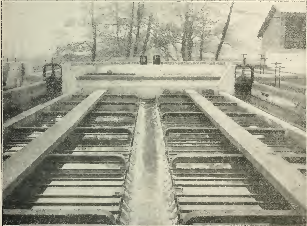
SEPARATOR AT STONE SEWAGE WORKS.
