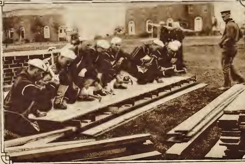
The Jackies themselves did much of the construction work. at Great Lakes.
