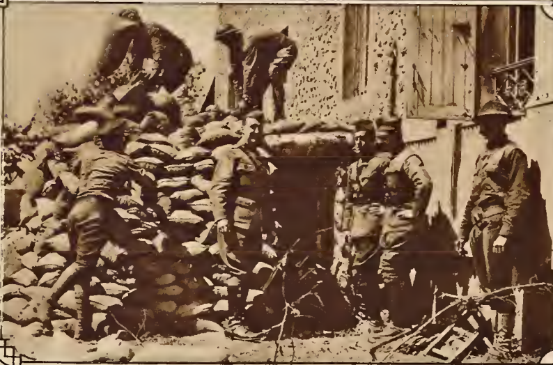
Col. McCloskey supervises the construction of a dugout at La Loge farm to be used as Marine and Artillery headquarters during the operations at Belleau Wood.
