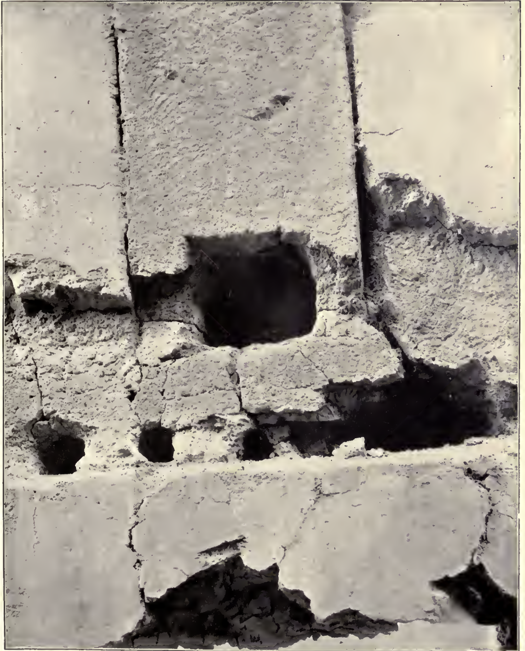
BLOCKED OPENING IN WEST WALL.
