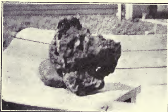
Photograph of One of the Rooms Showing Hardened Walls. A piece is broken out on one side.
