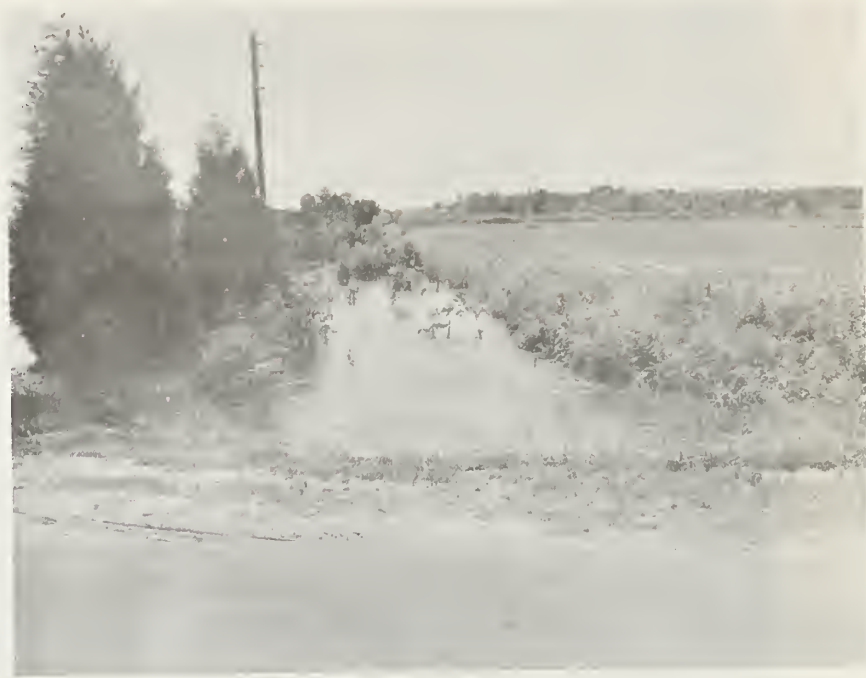
Lateral 1A at State Secondary Road 1312, culvert and inadequate channel restricts flow.
