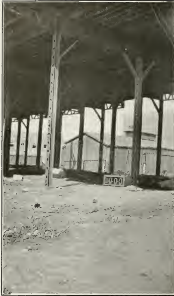
FIG. 49. WEST APPROACH TO FIRST STREET VIADUCT View of understructure, showing insufficient support.
