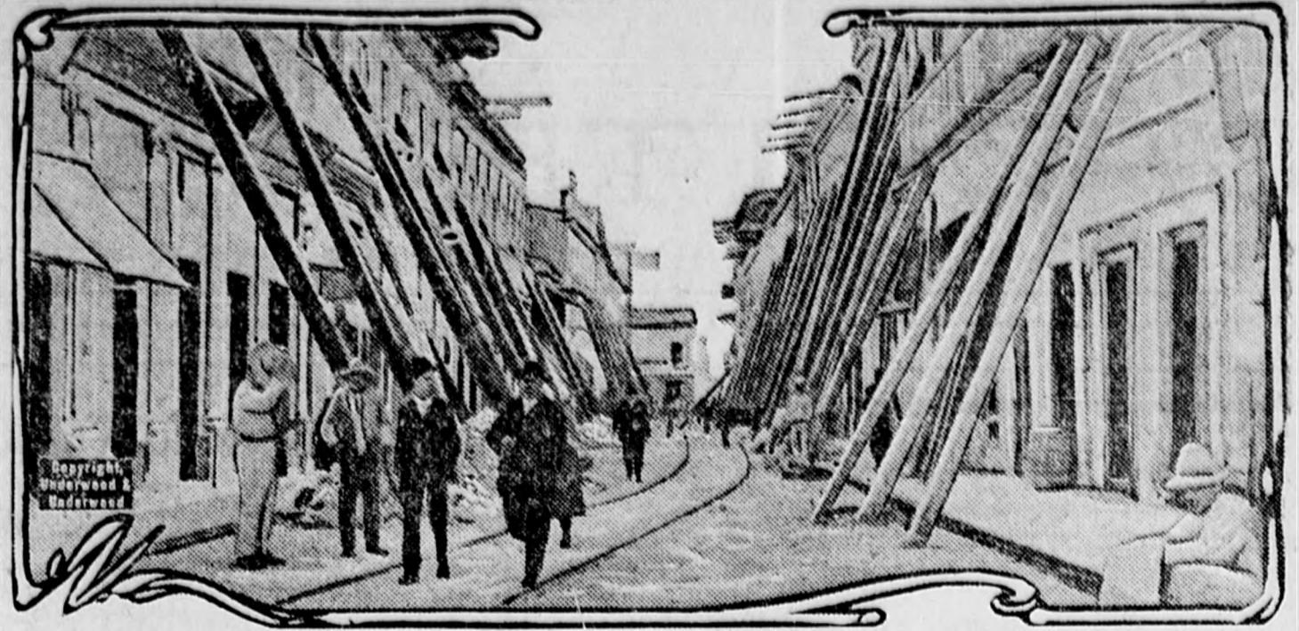
Buildings in Jalapa, capital of the state of Vera Cruz, Mexico, thrown out of plumb by the recent earthquake, are shown propped up to prevent collapse. Vehicular traffic has been suspended on the thoroughfares thus affected for fear the least vibration would bring the weakened buildings down.
