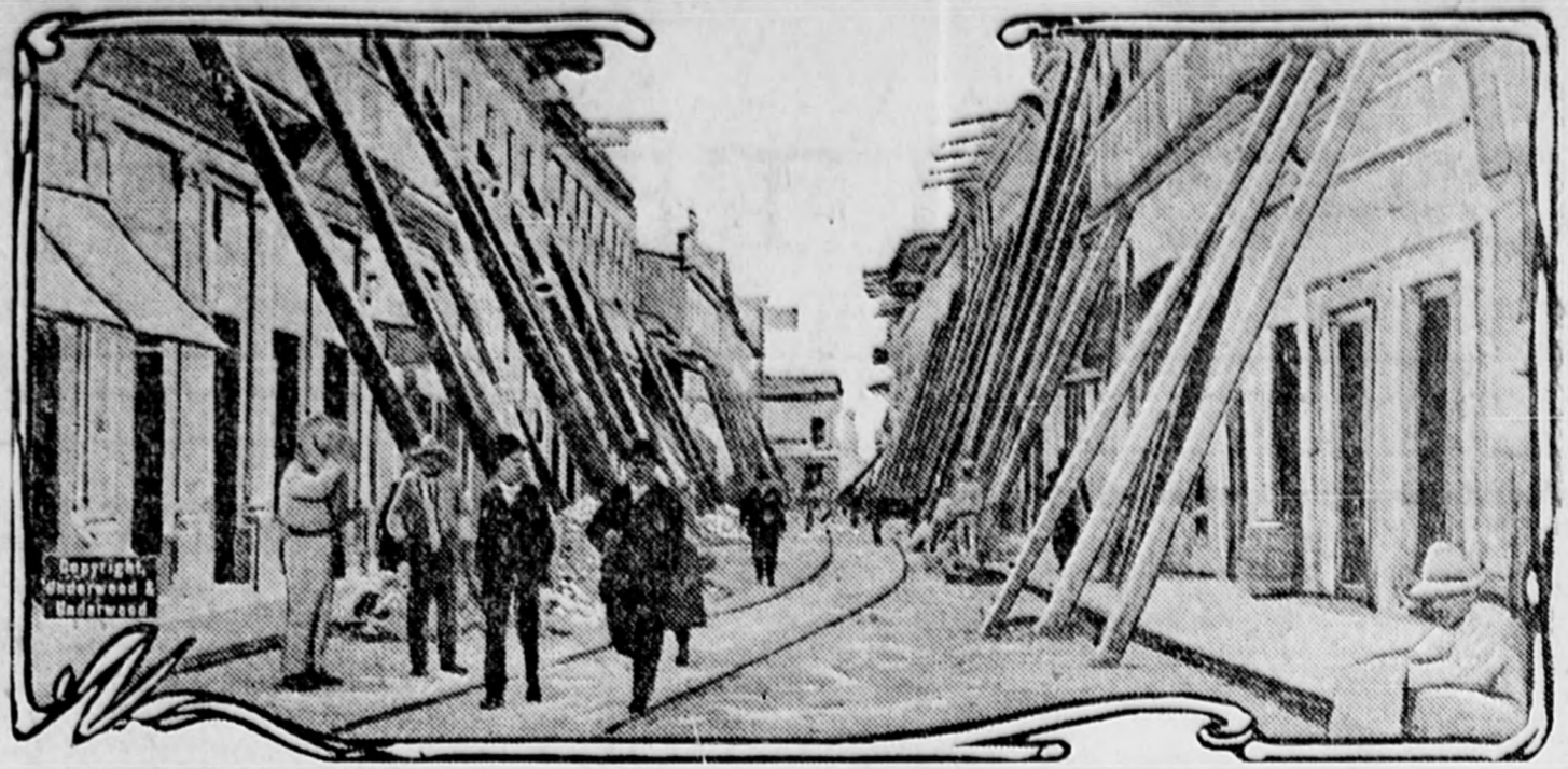
Buildings in Jalapa, capital of the state of Vera Cruz, Mexico, thrown out of plumb by the recent earthquake, are shown propped up to prevent collapse. Vehicular traffic has been suspended on the thoroughfares thus affected for fear the least vibration would bring the weakened buildings down.
