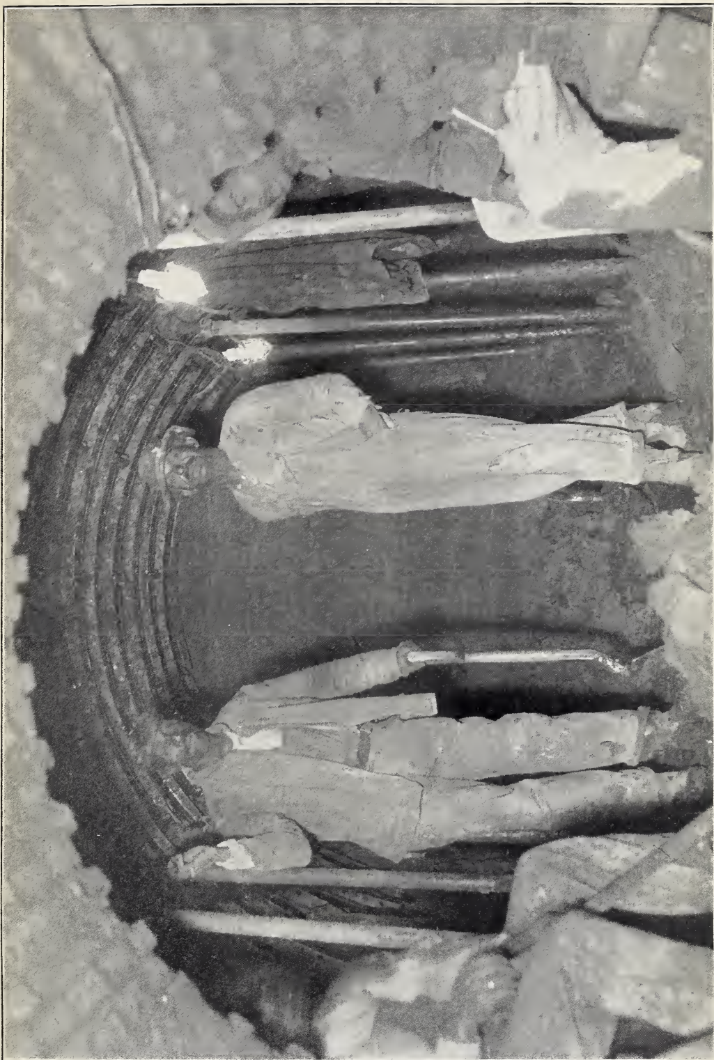
METHOD OF SUPPORTING ROOF PLATES IN TUNNEL HEADING—CONSTRUCTION BY COMPRESSED AIR ON HIGH LEVEL SEWER EXTENSION.
