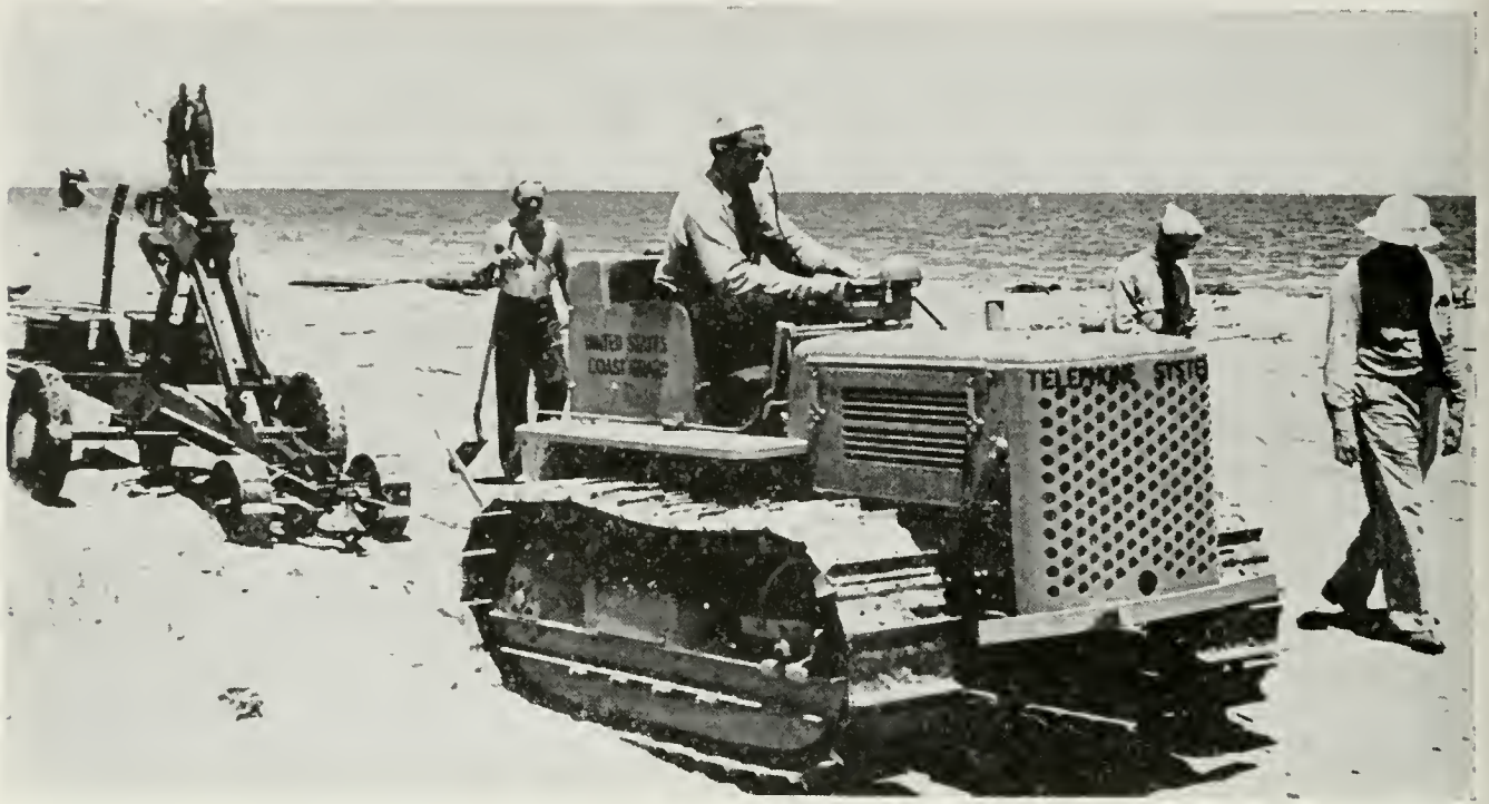
Plowing telephone wires into the beach for the use of Coast Guard beach patrols
