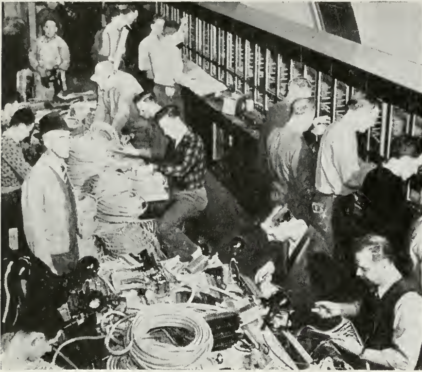
Inside one Quonset hut, installers are working on the first of three rows of switchboard positions which are being installed as fast as carpenters can lay the flooring
