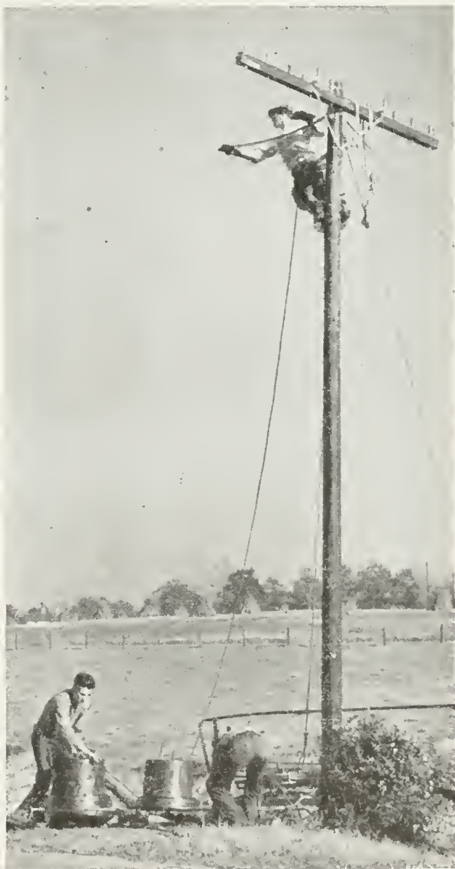
Then a long-span pole line is built to bring the high-strength steel wires into the neighborhood
