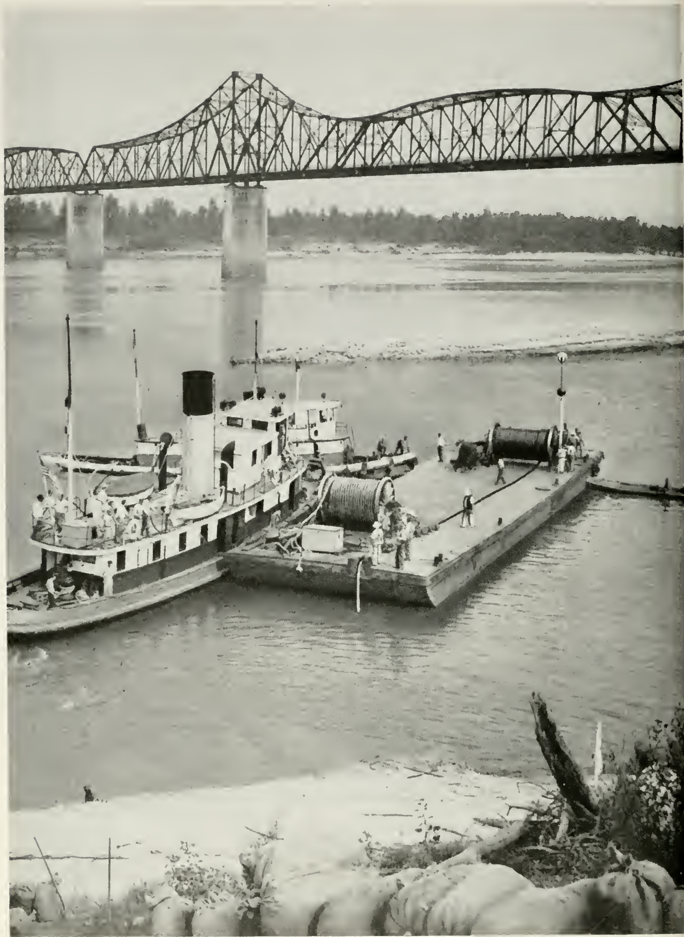
Crossing Ol' Man River: an armored section of coaxial telephone cable being laid on the river bottom near Vicksburg, Miss., as the southern transcontinental coaxial cable project pushes westward toward the Pacific coast. See page 147
