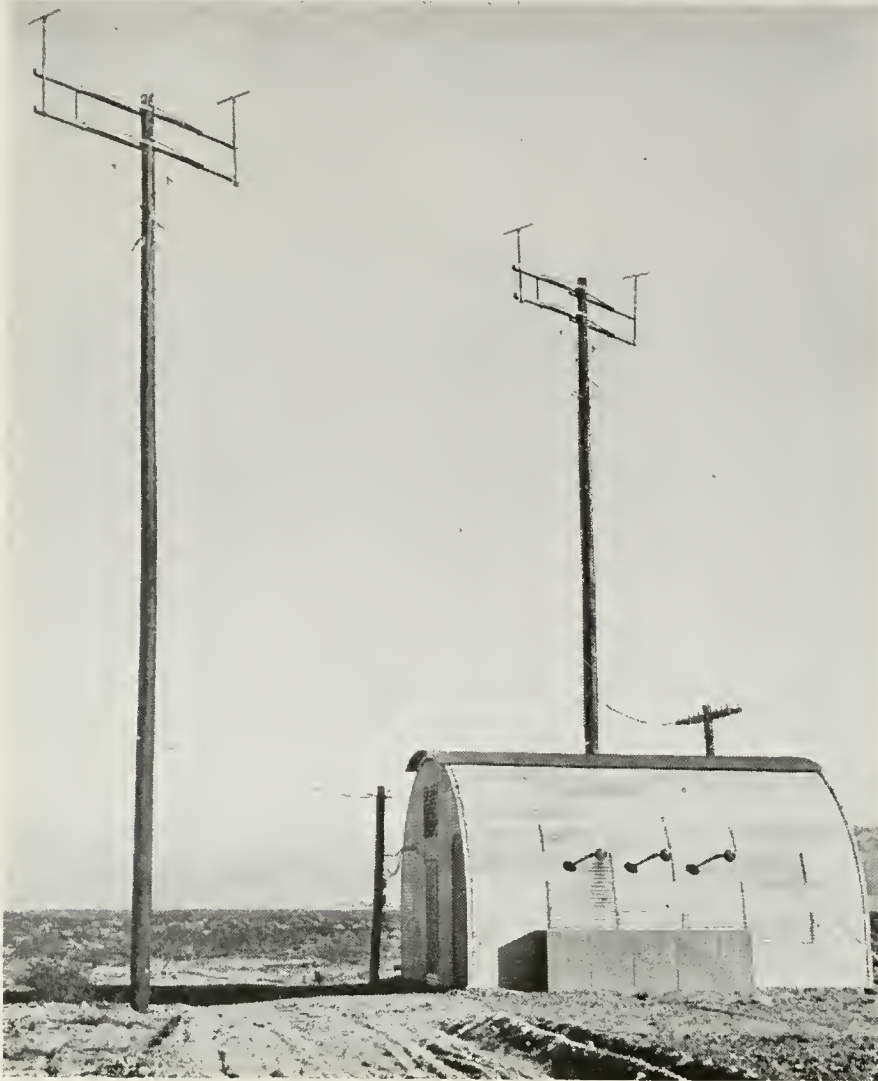
The antennas of the Death Valley terminal of the new radio telephone circuit loom over barren sands
