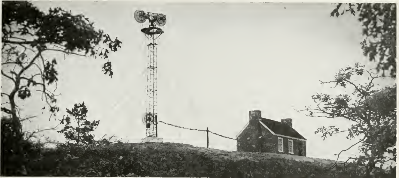
This recently completed micro-wave radio station on Cape Cod provides telephone circuits to Nantucket Island
