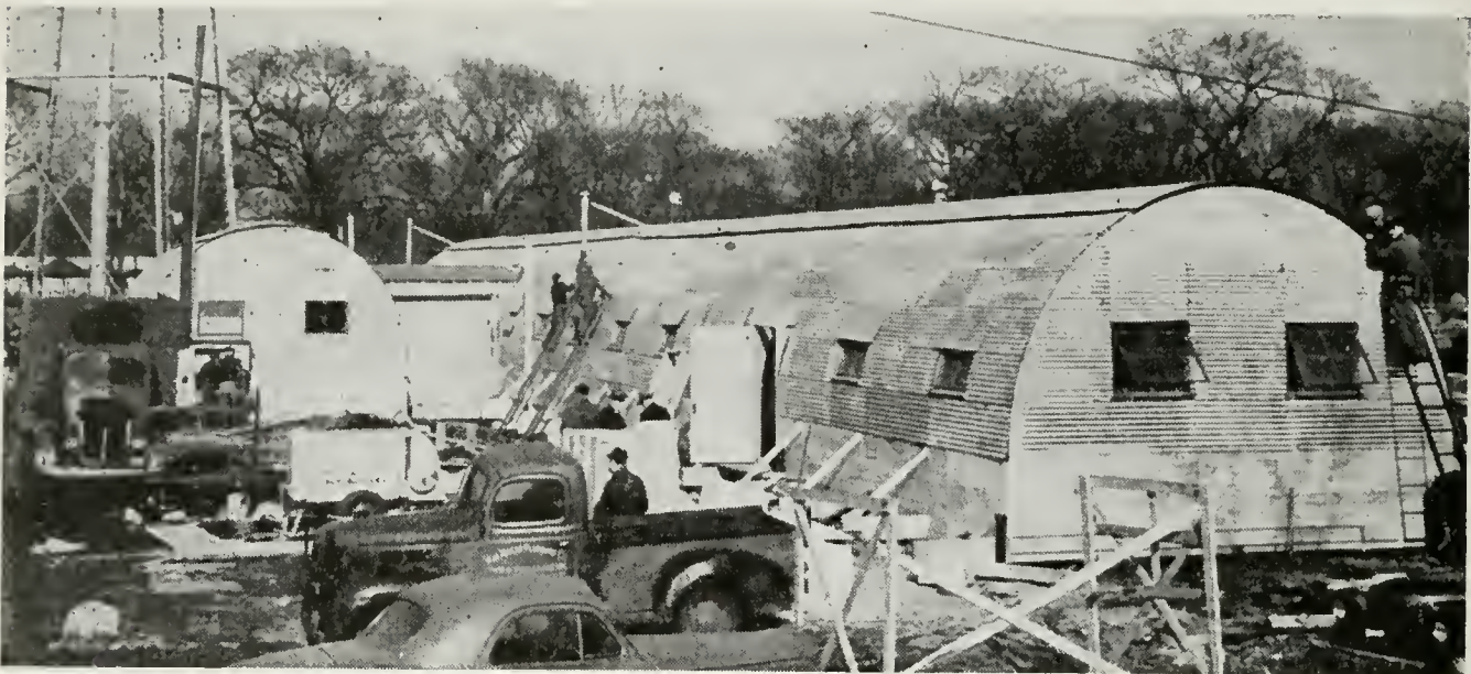
Equipment is going into these Quonset huts, behind the destroyed building, while the contractor's men complete the work of erecting them
