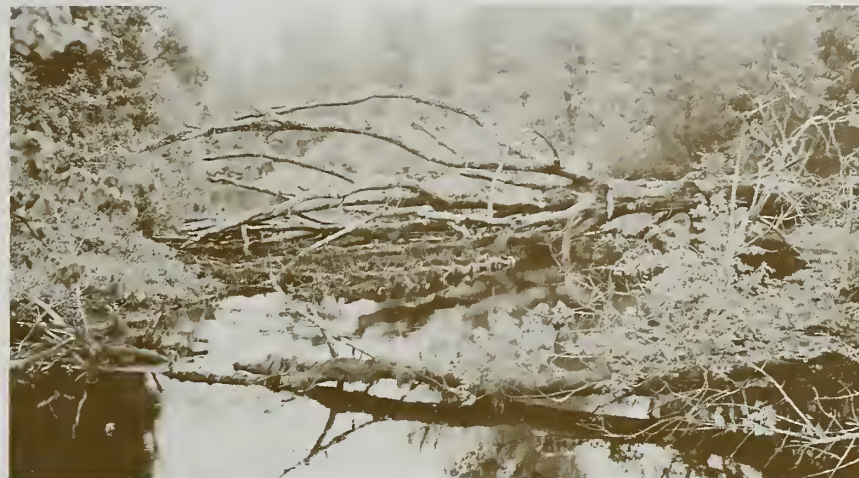
Windfalls clog the Pocomoke main creating temporary debris dams, thus causing a rise in normal water that restricts drainage for upland tributaries.
