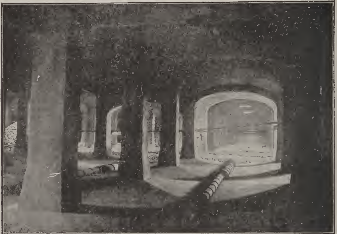
FIG. 122. — INTERIOR VIEW; WASHINGTON FILTERS. (From Trans. Am. Soc. C. E., vol. LVII.)
