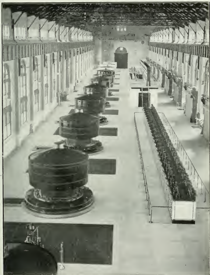
PHOTO No. 1504—Showing the Interior of Power House No. 2 of the Niagara Falls Power Co. at Niagara Falls, N. Y.
