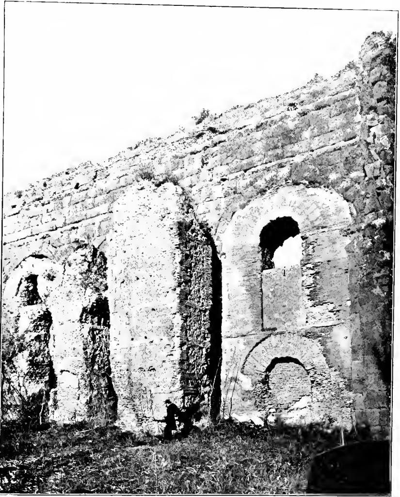
Claudia and Anio Novus near Porta Furba. Repairs in brickwork and in a composite of concrete and brickwork.
