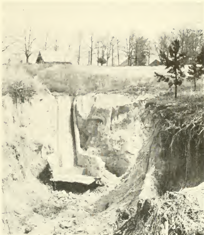
1. Damage due to an engineering construction planned without attention to geology and soil science.
