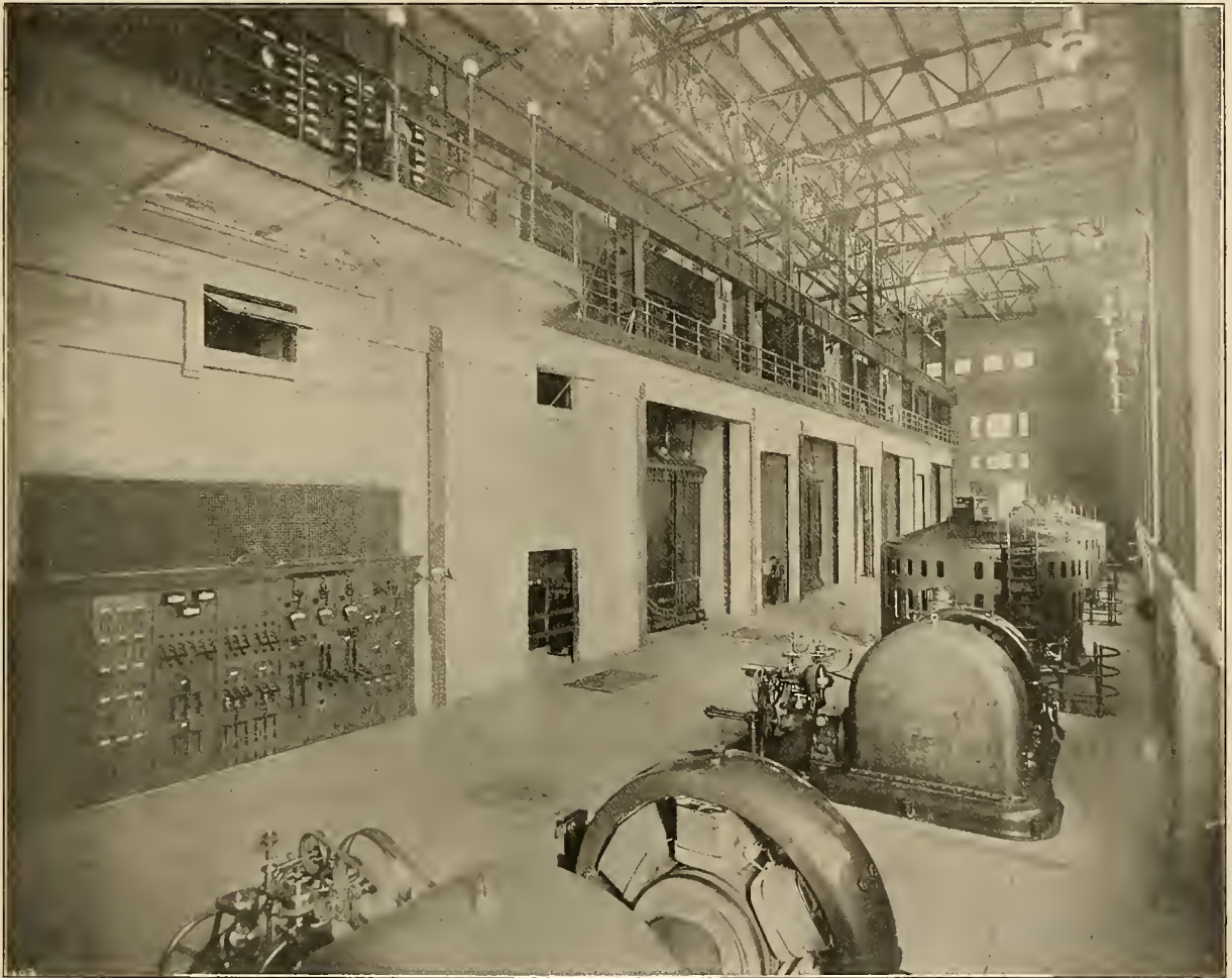
General View in Main Bay of the Powerhouse.
