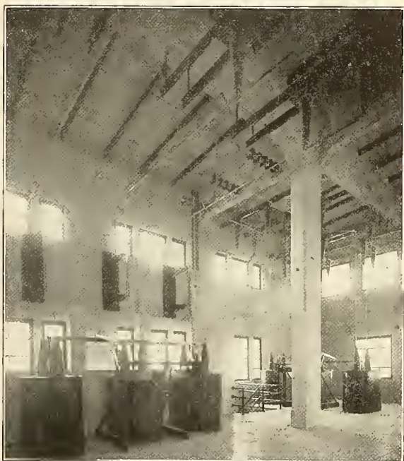
Incoming-line Oil Switches; Disconnecting Switches on Right. Transformer Oil Switches and Disconnecting Switches on Left; Brighton Sub-station.
