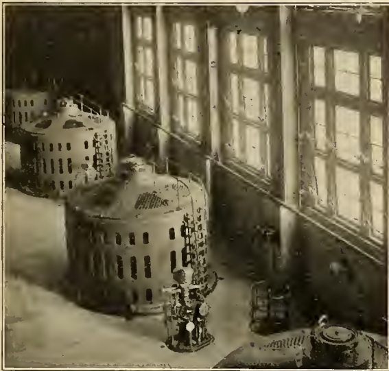
Main Generators and Governors.
