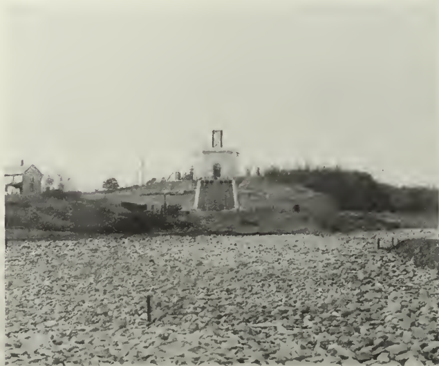
THE LANDSCAPE IMPROVEMENTS UNDER WAY. View from the south showing stone foundation for driveway and excavations for long water basin.
