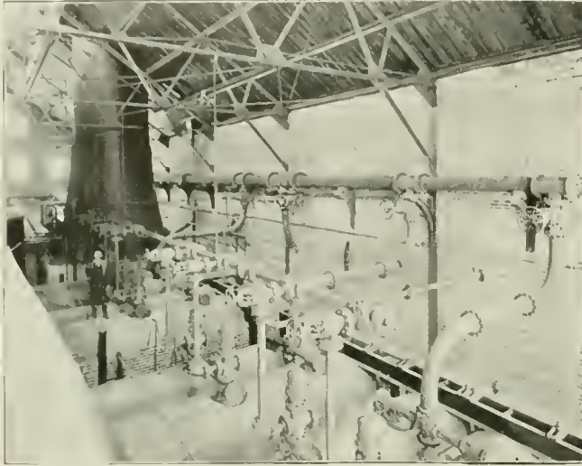
STEAM PIPING, KAW RIVER STATION.
