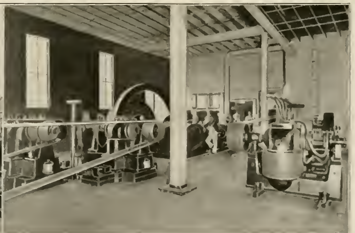
INTERIOR OF POWER STATION.
