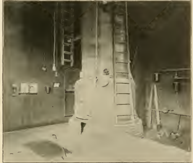
FIG. 1 BOILER IN FIRST POWER HOUSE.
