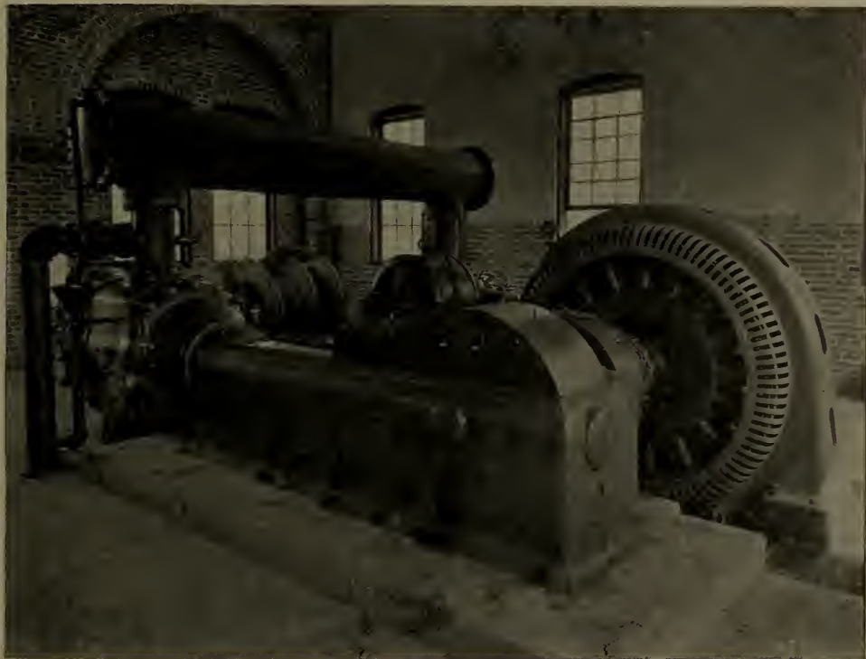
Ingersoll-Rand "Imperial XE" Duplex Direct-connected Electric-driven Air Compressor.
