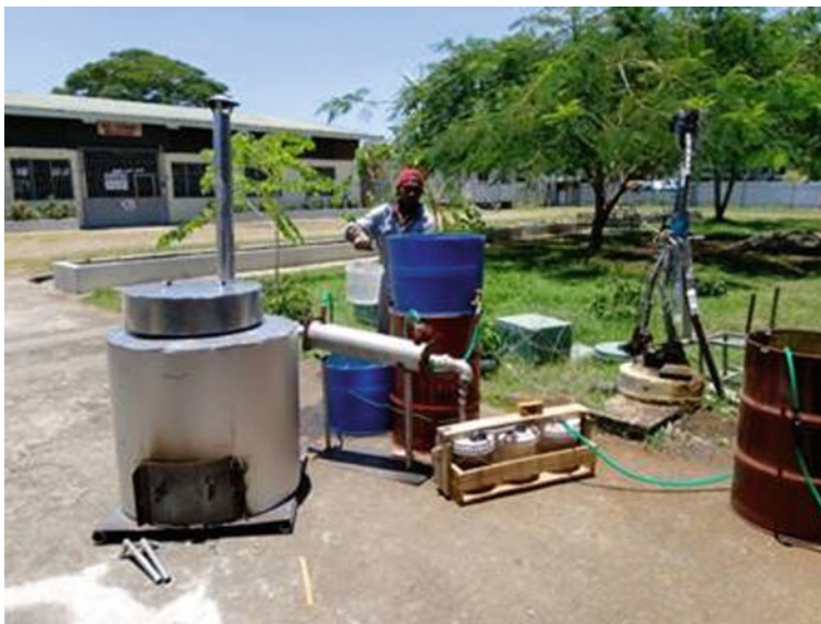
Fig. 18.4 Nufuels Ltd demonstration plant for plastic pyrolysis to produce energy in the Solomon Islands (©Nufuels 2020)
